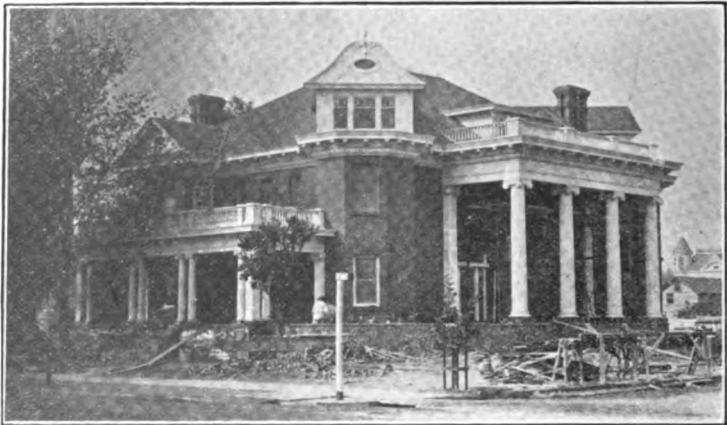
Residence of F. K. Prescott, under Construction, Fresno H. A. Hansen, Builder Fresno Brick & Tile Co., Brickwork
