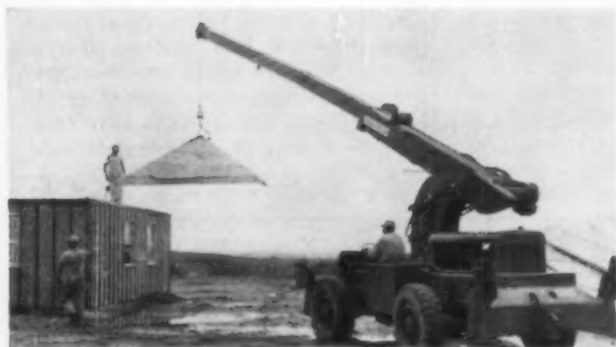
SMALL CRANE —Truck-mounted crane that extends and lowers hydraulically proves a versatile work horse handling components, pouring concrete, and doing chores on the job.
