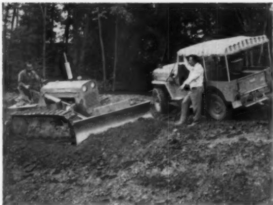
LITTLE RIG —Mears uses small International tractor with multi-angle hydraulically-operated dozer blade to trim dam sides and to do fine grading of sub-base for golf course at community-like Rustic Hills Development.
