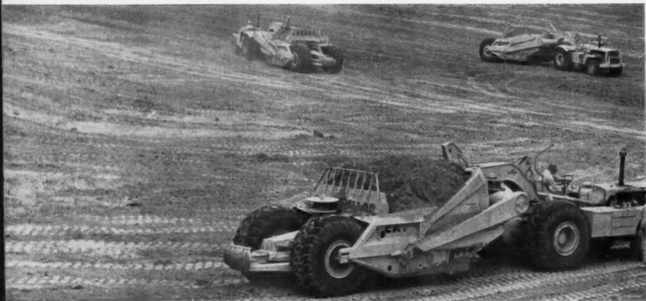
BIG SPREAD —Earthmovers belonging to Fischer and Fritchel of St. Louis haul earth on balanced terracing operation in an F&F
