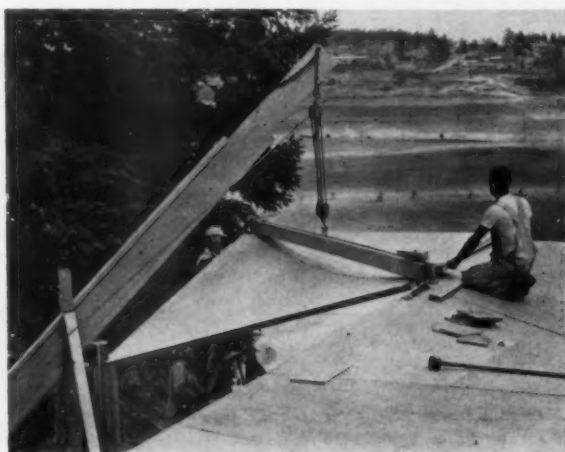
BOOM LIFTS roof panel on top of column (shown at left). When assembled, roof receives insulation and built-up roofing.
