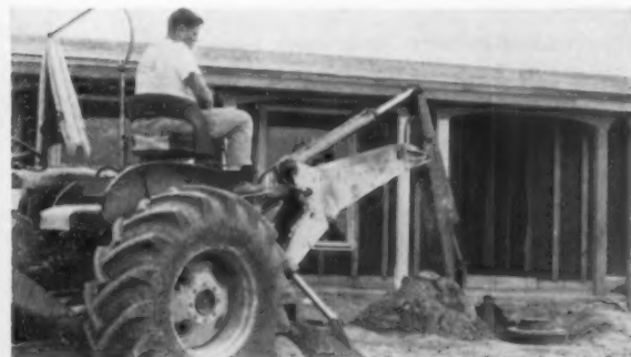
BACKHOE —F&F fits a small backhoe attachment to rubber-tired tractor to trench for power lines, sewers, and some foundations. Rig is part of a $250,000 fleet F&F operates.
