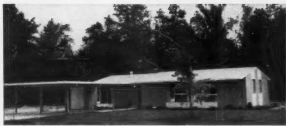
JOINTS BETWEEN PANELS are tongue and groove with panels nailed directly to framing members. Undersides are painted.
