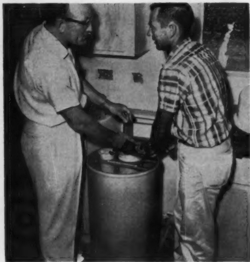
WITH BUILDER HANCOCK assisting, (left) unit goes under sink counter. Softener should be used on both hot and cold water lines, but should bypass all outside sillcocks.
