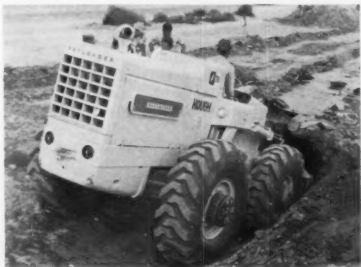
A LANDSCAPERS RIGHT ARM —Small Payloader fitted with front-end bucket tears up pavement for Arnold's Landscaping Company on a small service station job in Mesa.
