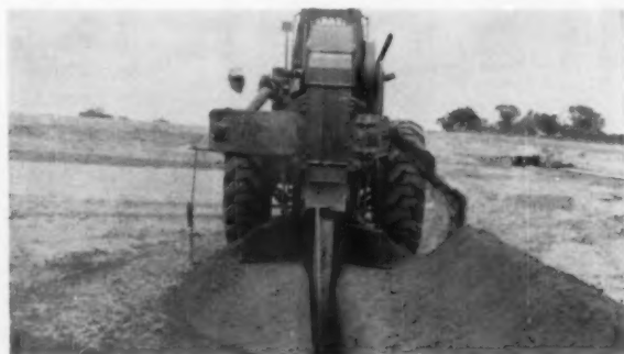
TRENCHER —Barber-Greene trencher fitted with a special flaring device cuts foundation trench and belled-footing simultaneously. Method enables F&F to pour four foundations a day.
