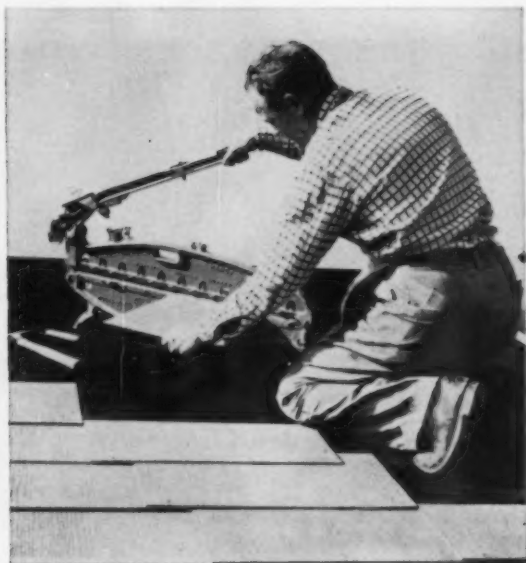
CUTTER on roof is used to trim asbestos-cement shingles for gable-end start—same technique as used with composition type of roofing material. Silicone treatment on the shingles—as siding—increases resistance to the weather.
