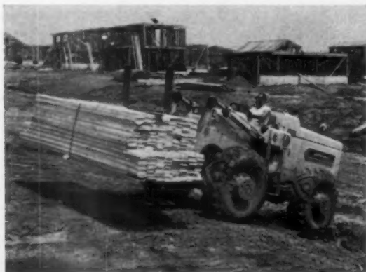
A PRODUCTION DREAM —Payloader fitted with modified lumber fork handles 1,200 bd ft of tongue-and-groove lumber on a 2,000-house subdivision known as Sayrewoods.
