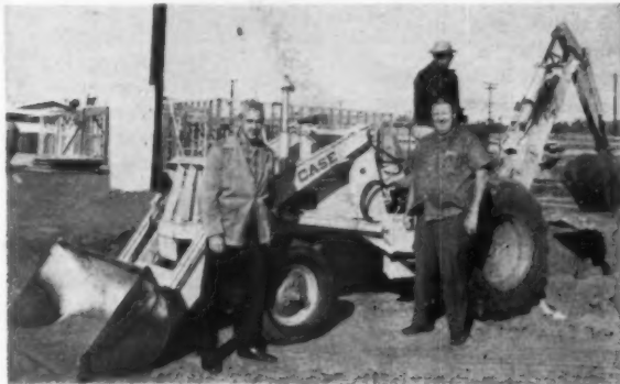
JOB PLANNING —Builder and equipment dealer plan next move for the versatile rig. Dune operates in a 50-mi radius of farm and desert country. Rigs move to jobs nearby under their own power. When jobs are far apart rigs are truck-hauled.
