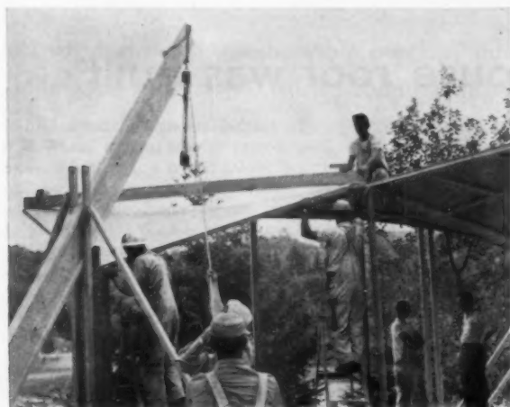
CONSTRUCTION VIEW shows light roof panel being positioned. Men on ladders align panel.
