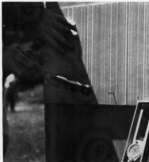
HAMMER, LEVEL , and cutter represent only tools needed for asbestos-cement work. Holes are already in siding—as well as shingles. Advantage of short lengths is ease of replacement should material crack or break.
