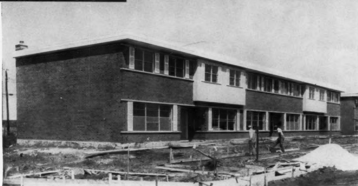
ONE OF THE LAST townhouses built in Quinn's project, this six-unit was sold out before completion. Homes are built on slabs.
