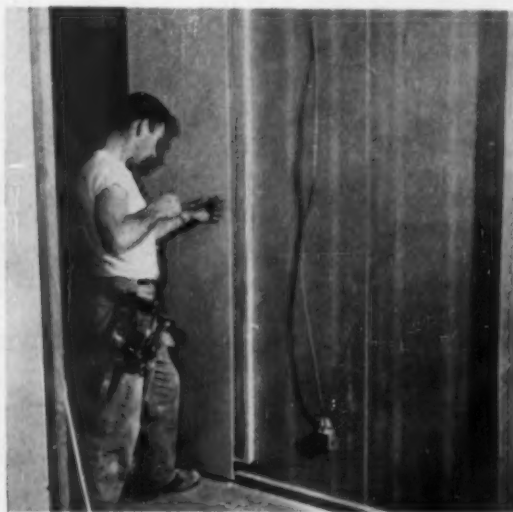
FINAL STRENGTH: insertion of flat head wood screw along edge of panel. Panels are applied to alternate sides of nailer strips, use 2x2 lumber for tracks.
