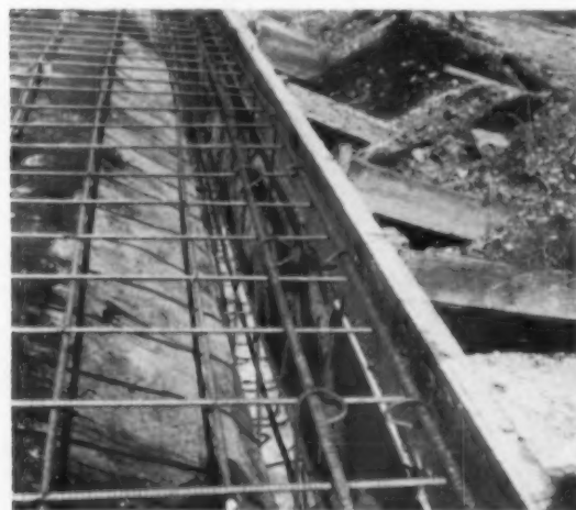
STEELWORK —Grid and exterior wall reinforcing consists of two 1/2-in. continuous rods to top and bottom, held together by 3/8-in. round stirrups on 15-in. centers. Slab reinforcing consists of 1/2-in. bars, 12 in. o. c., b.w.
