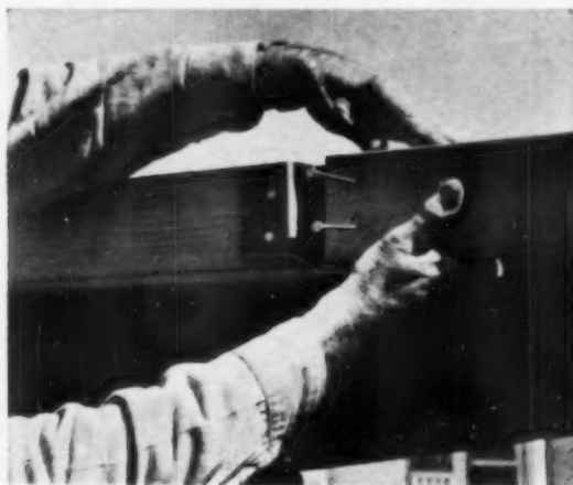
BUTT JOINT is used for fabricating roof, walls. As finish, some laminated walls are left exposed inside.
