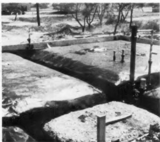
GRIDWORK —Trencher leaves a gridwork of concrete exterior walls and interior beams sloped to create inverted soup-bowl effect. All exposed surfaces are water-proofed with two layers of 15# felt lapped and hot mopped.
