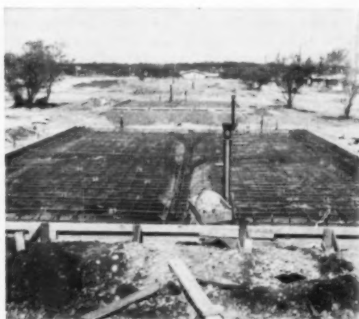
FORMWORK —Only a single perimeter form set on grade contains entire monolithic pour of concrete that will make up foundation. All plumbing, ducts, other fixtures are set into foundation base before concrete is placed.
