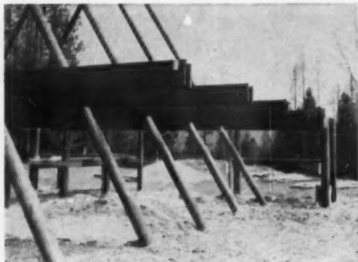
FLOOR BEAMS —double 2x10s—are spiked to poles. Beams support 2x4 outside, 2x6 inside decking. For accuracy of centers, holes are dug by augers, post-holers.
