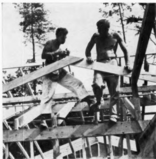
CLERESTORY LIGHTING is unusual feature (see above). Insulation batts go between 2x8 "rafters."
