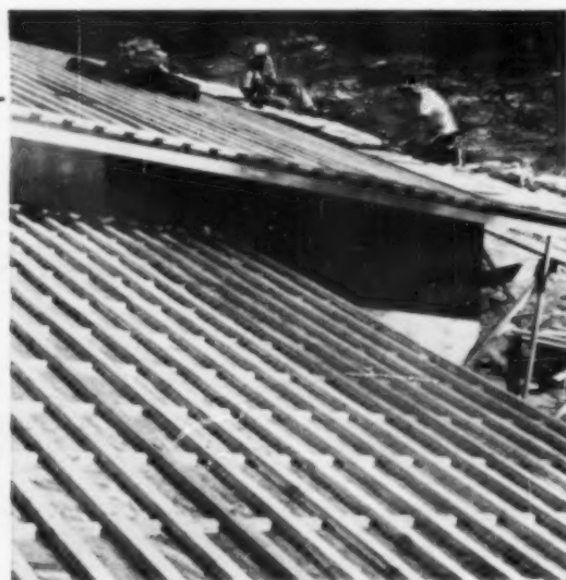
FRAMING permits air circulation between sheathing, shingles. Edge of roof above fascia is left exposed for this.
