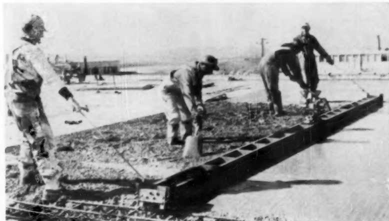
GAS POWERED 28-ft. Thor vibratory screed is pulled across a section of ceiling slab. Underside of slab will be so smooth that it won't need plastering.
