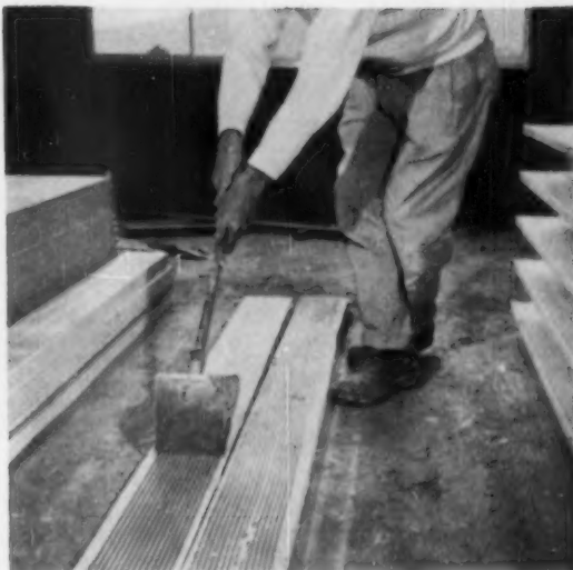
SOLID GYPSUM RIBS are laminated between sheets of Kaiser's Quilt-Lok wallboard to form wall panels. Laminating compound is spread to an eight-inch width.
