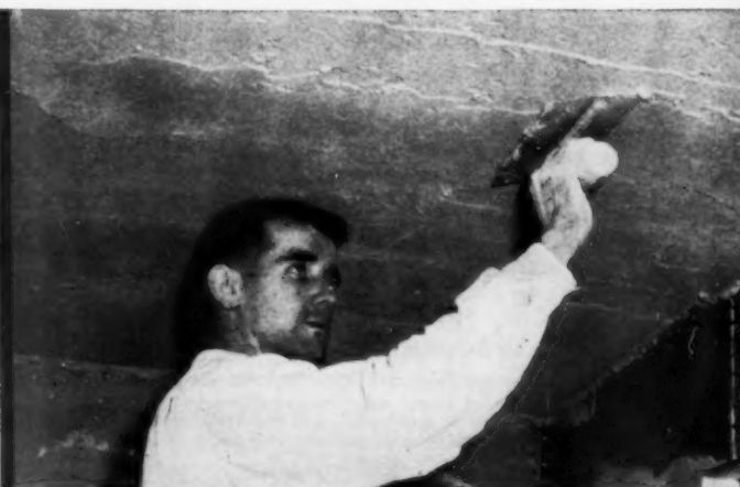
Plaster is applied over reinforced ceiling. The open mesh of both Keymesh and Keycorner assures imbedment in plaster. The open mesh also insures full bond of plaster with gypsum lath.
