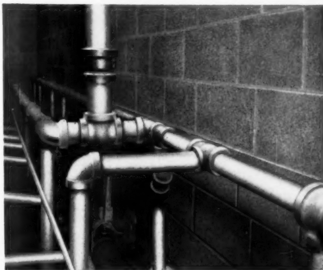
Proof of the integrity of galvanized steel pipe for drainage and vent lines is illustrated by its selection for so many modern new buildings, as in this installation at the great New York Coliseum.
