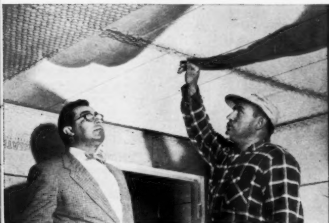
Eby (left) inspects application of Keycorner, used to reinforce joints. Keycorner is also used at all wall and corner junctures.
