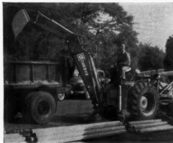
In Seattle, Mr. Sam English, one of the owners of Excavators, Inc., reports a saving in money on a utility contract because the Sherman undercuts eight feet unbroken sections of pavement, thus eliminating expensive handwork. He says, "The maneuverability, efficiency and economy of the Sherman make it the best digger I have seen."
