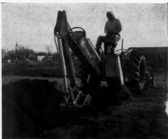
Mr. L. L. Donaghue and Mr. Vernon O. Lippoldt, co-owners of the D & L Ditching Service of Haysville, Kansas, say, "The Model "F" is our fifth Sherman digger and if we were going to buy a digger tomorrow, it would be one just like this one. We already have 275 hours on it and have yet to tighten a bolt."
