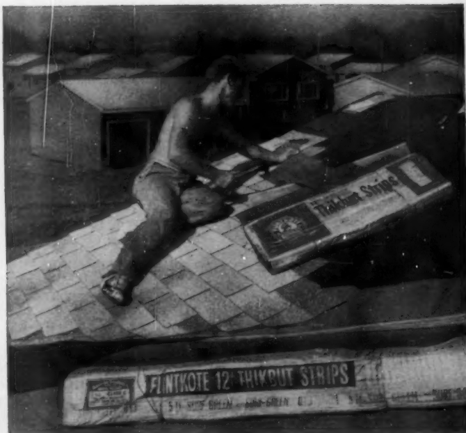
FLINTKOTE Thikbut 12" Strips go on in jigtime. The interesting colors harmonize with and set off the FLINTKOTE Asbestos Siding on houses in this fast-selling New Jersey development.
