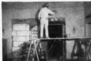
Ambassador Hotel, Milwaukee, Wis. Need for new washroom caused lobby wall to be broken through. Plaster-Weld was applied to old surrounding painted wall to facilitate blending of white coat from patch over old wall. One of many applications for this versatile bonding agent. General Contractor, Kurtischenreuter Company; Plasterer, L. W. Rosin.
