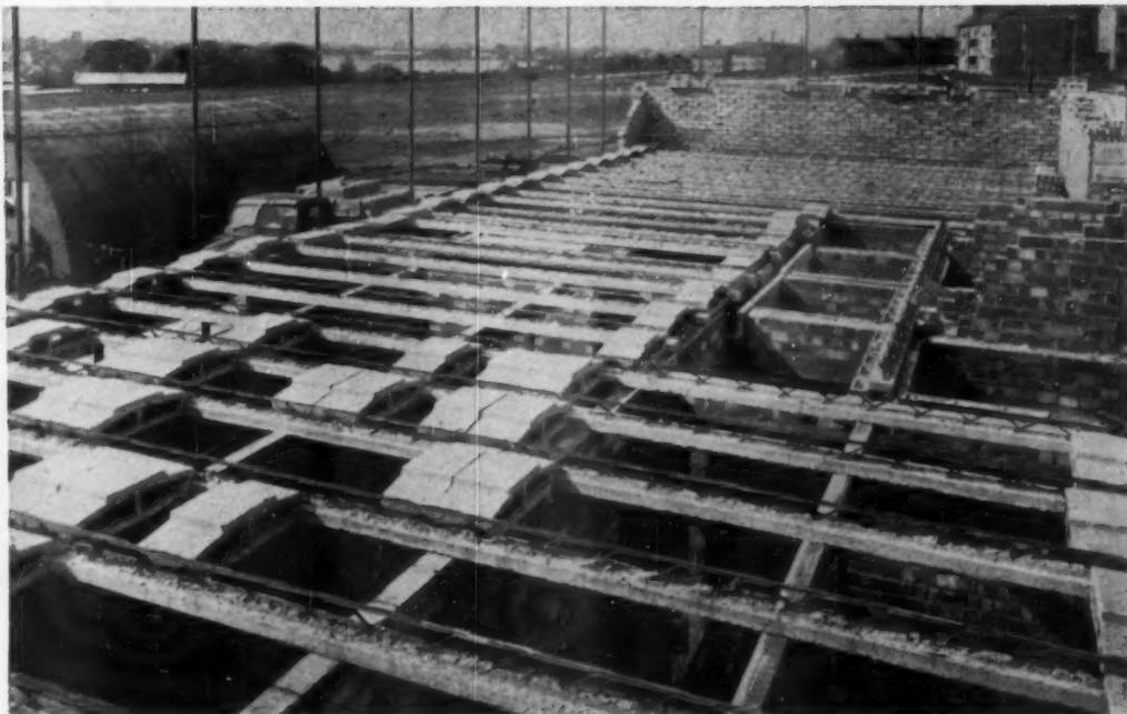
WOOD BEAMS supported by jacks, mid point under concrete blocks and Omnia planks, aid in leveling floors.
