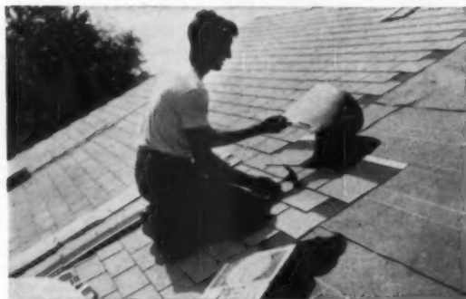
WIGGINS BROTHERS , Charlotte, N.C., will receive hurricane protection from Flintkote Company's award. Prize, for good merchandising of "Hidden-Values", is "Seal-Tab" shingles for a whole roof job.
