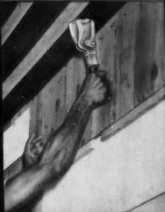
Speed undercourse shingling with H2B Hammer's one-hand, one-blow operation. A foot longer reach!
