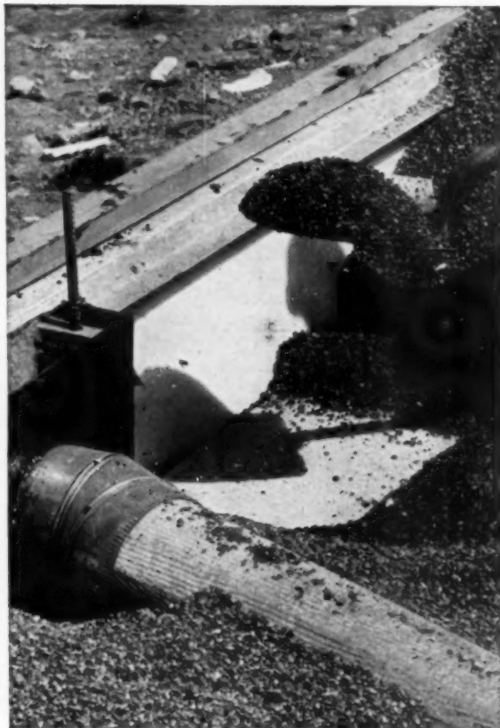
2. Styrofoam insulation 1" thick is then placed at an angle 12" high against the poured foundation wall.
