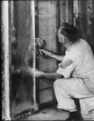
Tacking foil insulation to face of studs is fast, neat and secure with the H2B Hammer.
