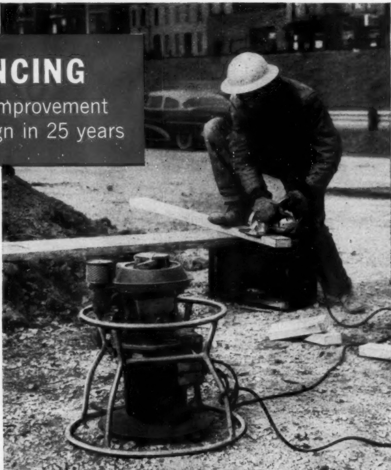
New Thor generator powering a Thor 7 1/4" SpeedSaw hastens construction of the new Congress Street Expressway in Chicago.
