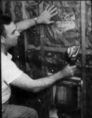
Metal lath goes up faster, with less effort, when one hand positions lath on studs, other drives staple.
