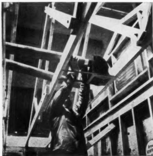
A FURNACE has been installed at front of house. Here a new type of duct, insulated with fiber glass, is connected to a warm air outlet in the ceiling.
