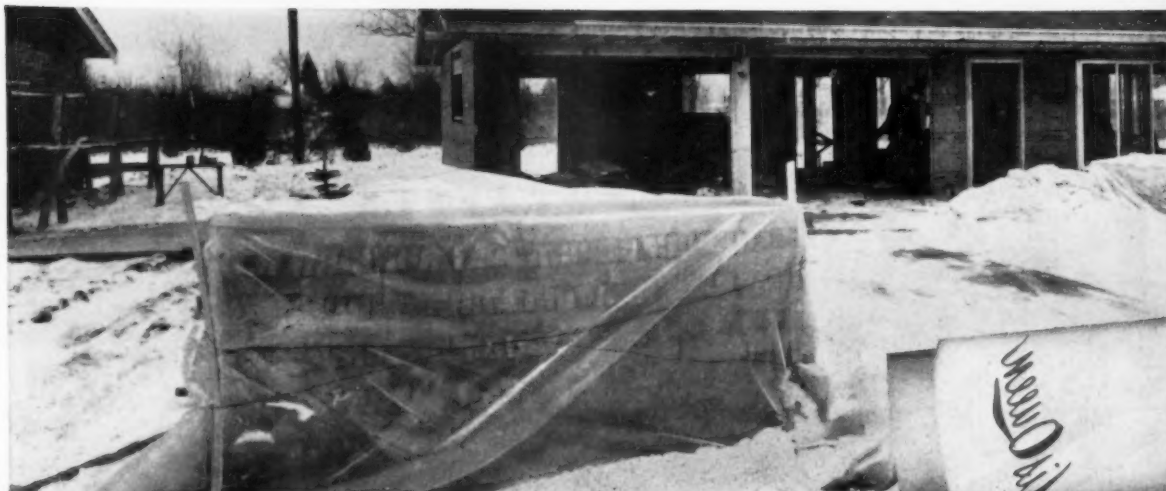
Notice all the on-the-job uses for VISQUEEN film at Braun Builders present site in Saginaw.
