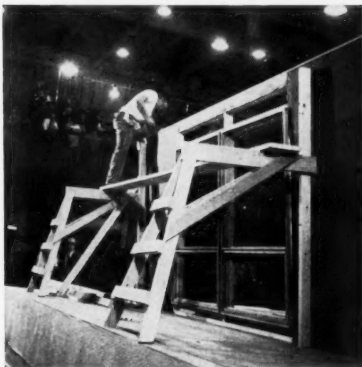
C OPPOSITE WALL PANEL has been tilted up and is held in position by scaffold horses. Window frames are nailed directly to studs, cripples eliminated.
