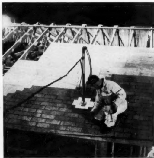
B MAST for electrical service is run up through the overhang, meter panel is set on wall below. This is as far as the roof sheathing and shingling went.
