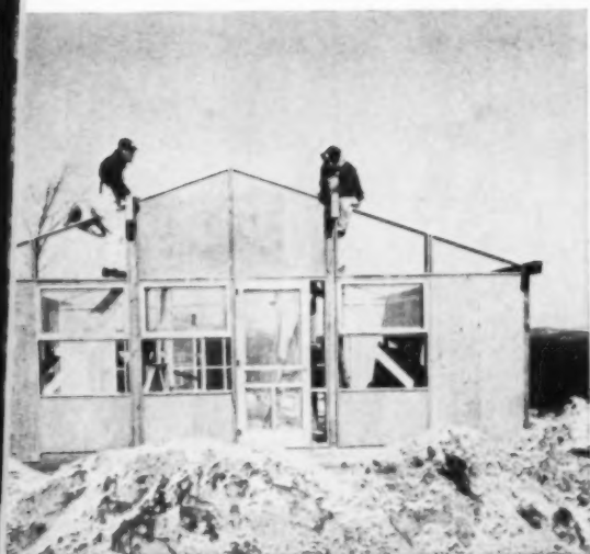
CENTER PANEL OF GABLE END is dropped into place. Modular structure is clearly shown in this picture; nine panels and two 4 x 4 posts make up the entire front of the house. Girders extend to carry porch roof.
