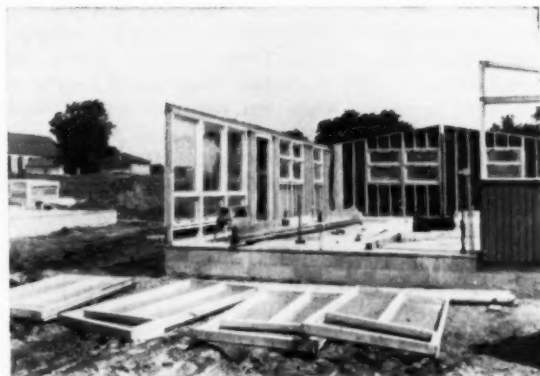
Costwise, the Lu-Re-Co system beats conventional construction. Young Schaub can erect the panels for a house in one hour and 20 minutes with a crew of four men
