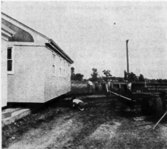
SECTION ROLLS on special rig for transportation to site. Transportation costs are $110 for the first 25 miles
