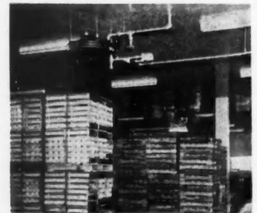
UNIT HEATER shown in a portion of the company's warehouse. Steam is fed to these distribution outlets from two large boilers in the basement of building
