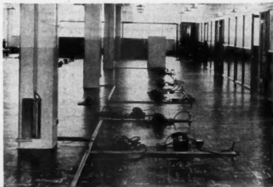
INSTALLING telephone service for offices in surface raceways brought about considerable saving in remodeling costs
