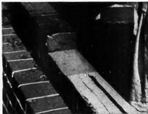
A good bond was not secured here because the brick on which the mortar was spread had sucked the mortar dry, before the brick was laid.
