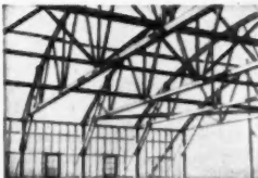
This shows construction detail of 71' 10" by 70' hangar erected at Holman Field, St. Paul, Minnesota. Trusses are spaced 10' O.C.
