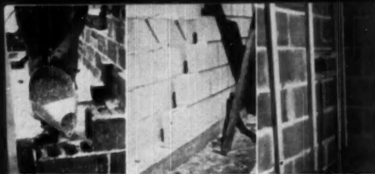
FILLING block with granular insulation, building hollow double walls, and applying lathing strips for interior finish are three ways of supplementing masonry insulation
