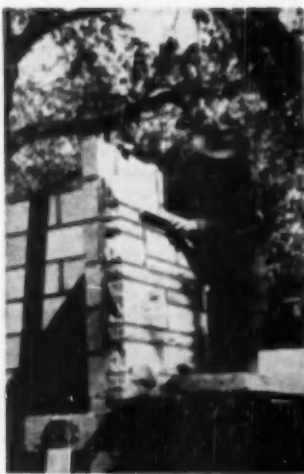
CONCRETE masonry slabs, four inches thick, are being used above, as back-up for window. Mason is tooling the joints
