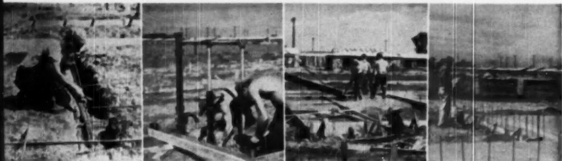
LEFT to right: Trenches for footings are dug the first day construction begins on a Martin Gunite home. On the second day,
