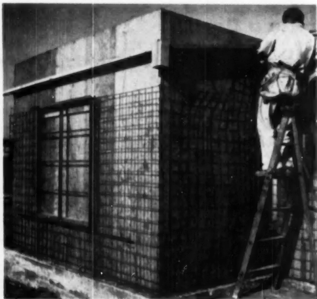
STEEL 4x4-inch wire mesh is placed in center of wall spaces and secured to dowels in slab before Gunite is shot against plywood forms. Note reinforcing around steel casement.
