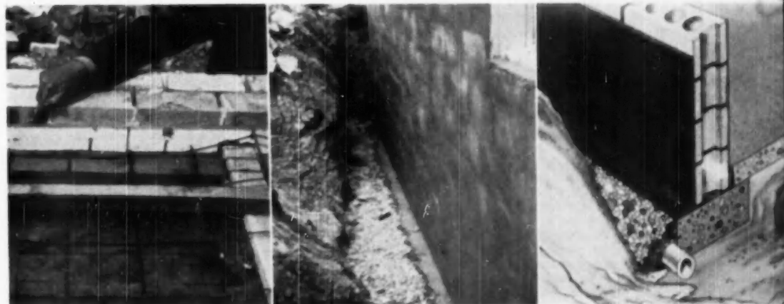
A ONE INCH barrier between concrete floors and walls is essential to reduce heat losses. The middle photograph pictures a basement wall coated over footings with coarse fill over tile. Diagram shows waterproofing cross-section
