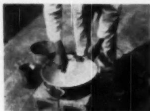
1. THE powder is added to the water and intensively mixed before applying to walls
