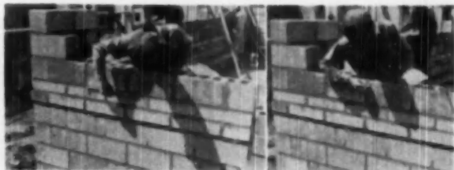
STRIKING joints serves two purposes: Accenting horizontal lines produces pleasing architectural effects. Sealing the joint with a tool helps prevent leakage
