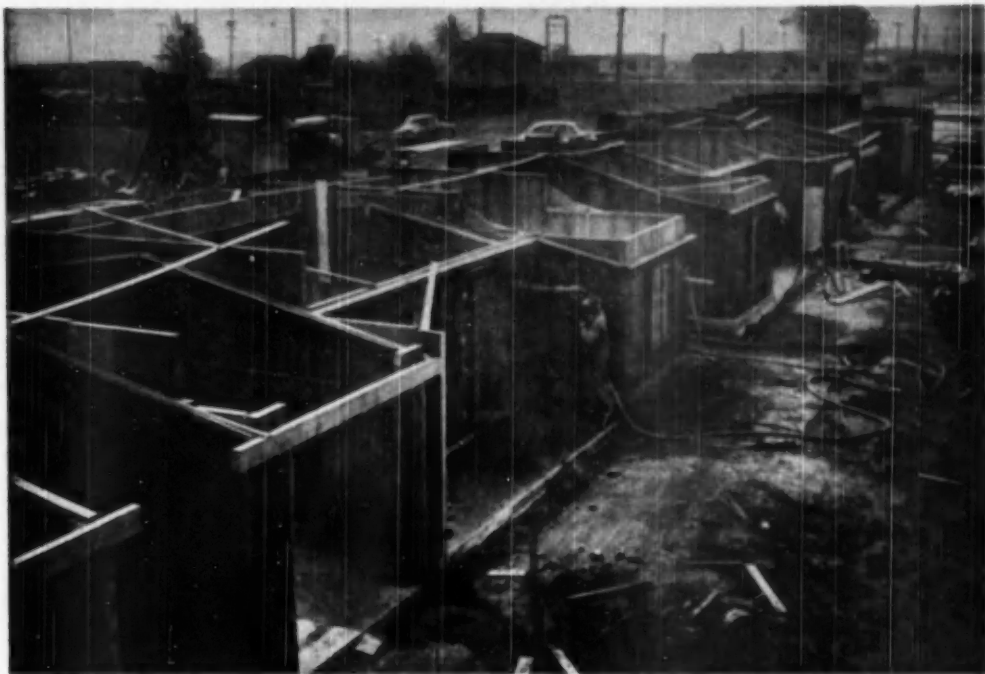
GUNITE, with Rochlite aggregate for insulating qualities, is "shot" on to form 5-inch walls in Arthur E. Martin project
