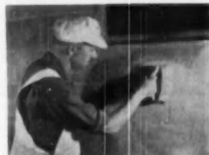
5. VIGOROUS brushing is necessary to insure that all openings in wall are coated
