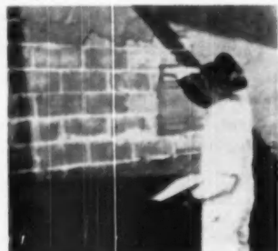
MASONRY units form good base for stucco, applied in one direction to prevent dry edges. Clean walls make best bond.
