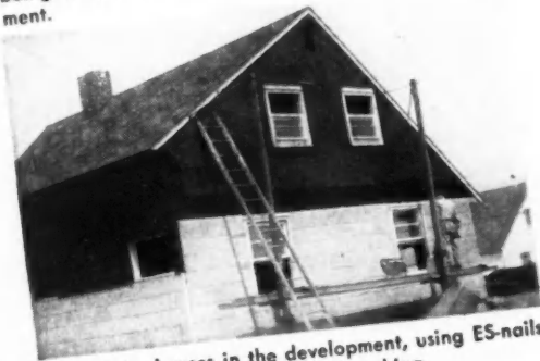
A portion of Levittown, Long Island, showing houses being completed in this tremendous housing development.
