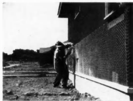
Keymesh being applied to side of house. Note how it unrolls flat—no bulging or sagging.
