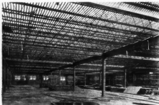
Interior construction view of new Westinghouse Corp., office building, Los Angeles, Calif., showing Truscon Steel Joists in place. Kaufman, Lippencott & Eggers, Architects. T-S Construction Engrs., Inc., Cont.
