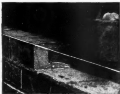
When mortar is spotted on only one corner of the brick, slushing seldom fills the voids.
