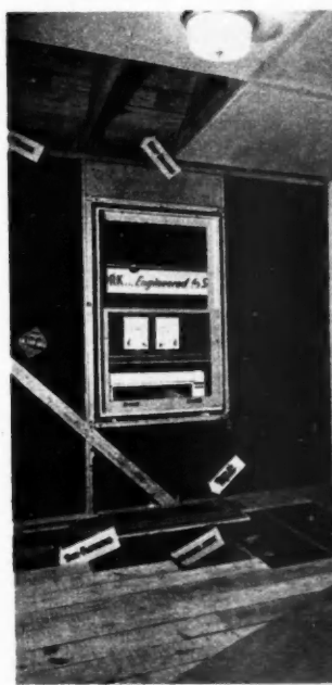
INCOMPLETE bedrooms show construction methods used, materials from which house was fabricated
