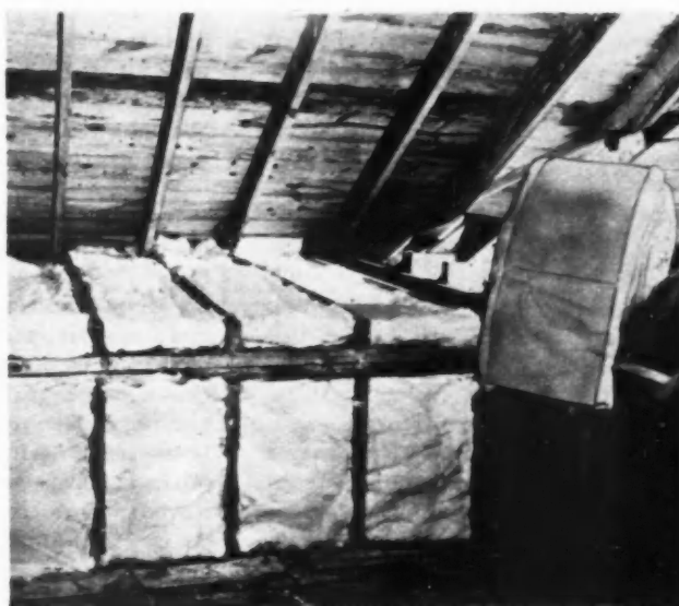
6. COTTON insulation installed over entrance hall. Resilient cotton has regained its original fluffy thickness
