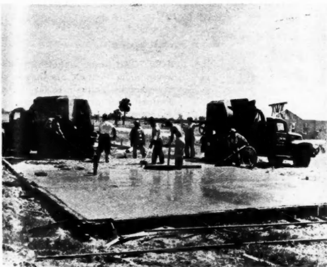
MONOLITHIC slabs and footings are poured and finished in an operation using reversible forms. A one-piece aluminum template is used to locate anchor bolts in slab. Rough plumbing in place
