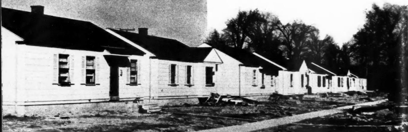
A FEW of the partially completed three-bedroom economy houses in one of the projects of H & L Builders
