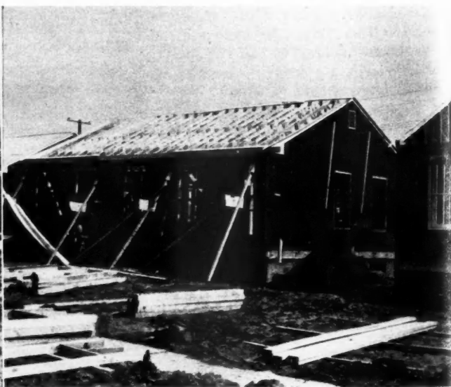
FRAMING for openings is assembled and delivered to framing crew which nails up wall sections on the boxed foundations
