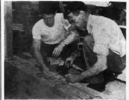
PREPARING to insert a thermocouple in the wall of the Maumee dwelling. Temperature records will be kept of a period of months.
