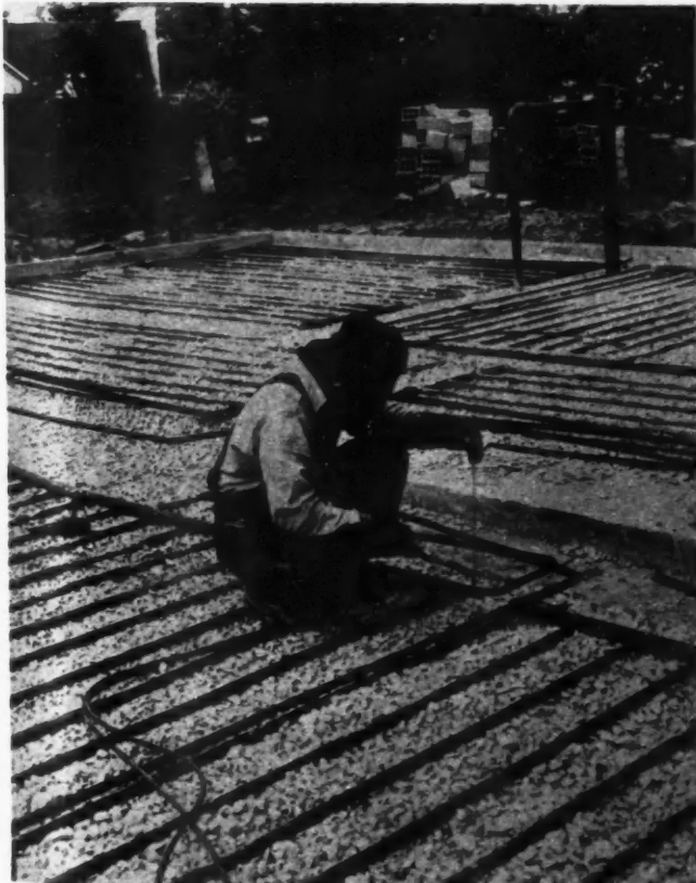
WROUGHT iron piping for radiant heat is welded on the job site.
