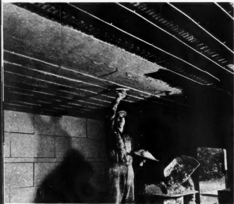
WHERE copper pipe is used it is imbedded in the plaster as shown.
