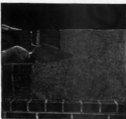
Or if the back-up units are laid first, the front of the back-up units should be plastered in the same way.
