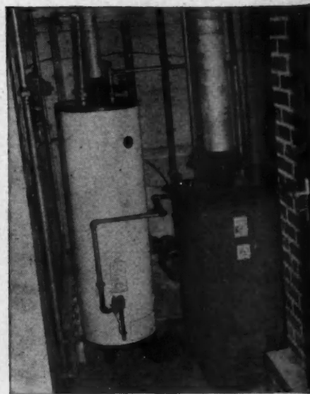
VIEW of compact gas fired heating plant.
