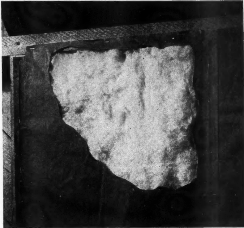
Up at the top of the studs is where many insulation jobs eventually fail. The normal vibration of the building causes many insulation materials to settle and pack down, leaving a heat-wasting gap.
