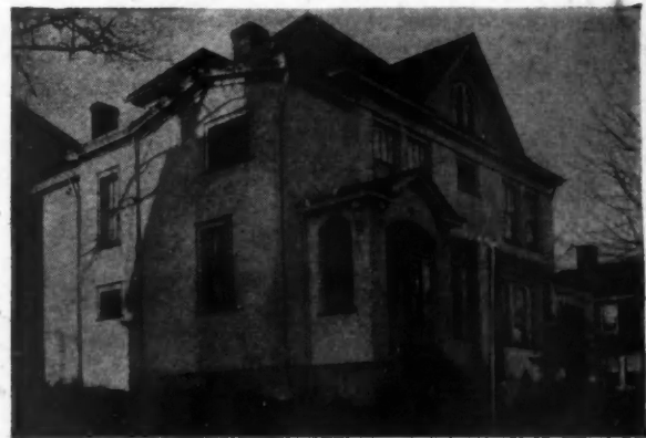
The above photograph shows the same stucco home after it received one heavy application of THOROSEAL, which, after being applied for one year, shows no leakage or dampness on the interior of the building.
