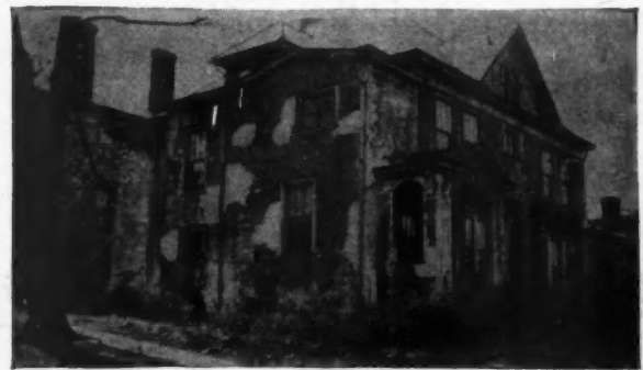
An example of disintegrated stucco surface on an otherwise well-built home and how the stucco was sealed, waterproofed and interior of home made dry with one heavy application of THOROSEAL.
