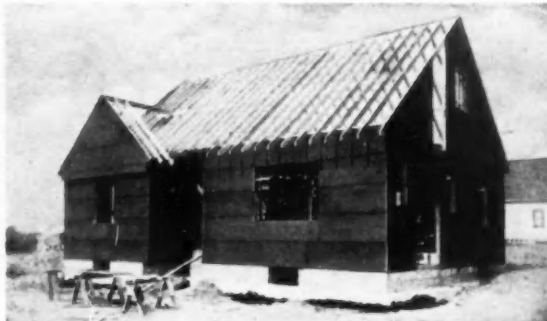
CUTS SHEATHING COSTS 1/3 TO 1/2. Cut and nailed right on the studs. In an actual job test 1,504 sq. ft. of this sheathing were applied in eight man-hours. Each unit is 2'x8'x 1/2", can be easily handled by one man . . . practically no waste.
