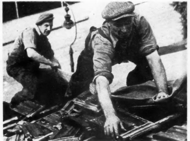
ABOVE: On the roof of a house they drag the tarpaulin over damaged and missing tiles, keep out the July summer rain.
