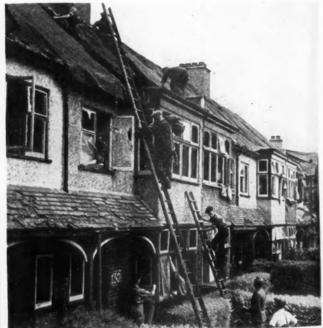
ABOVE: Typical of the damage done to house in the near neighborhood of an exploding flying bomb. Tiles are off the roof, windows blown in. The building army gets to work with tarpaulin and waxed linen "windows."
