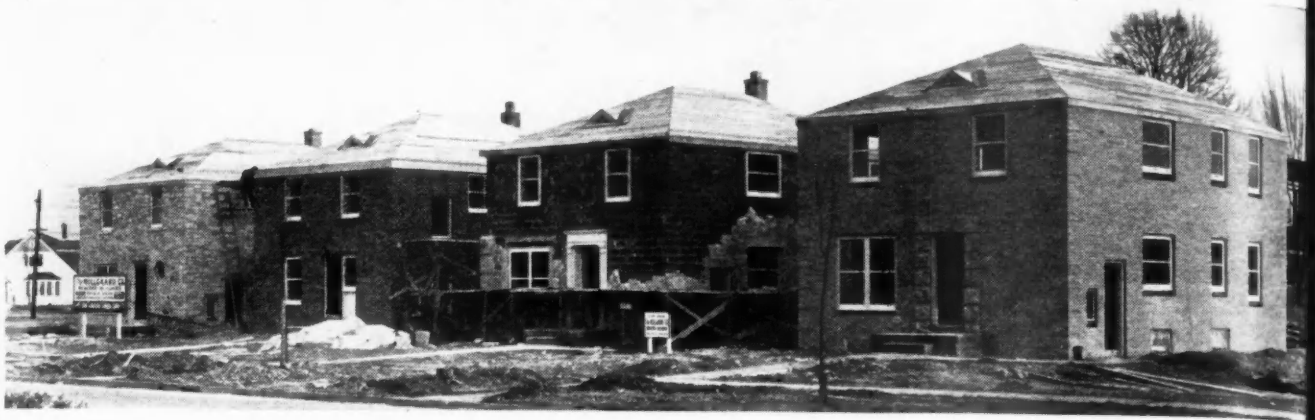
STREET of Milwaukee two-family war homes now under construction by builder Mollgaard.
