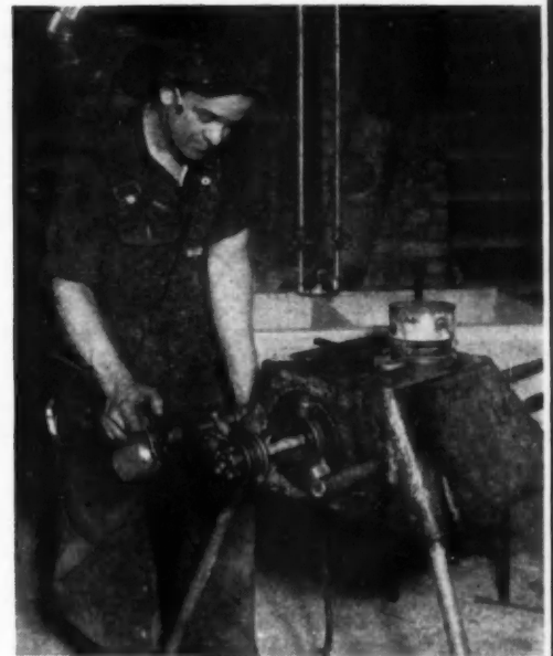
LOWERING erection costs of a job is a matter of reducing the time element in every way possible. At the right is a pipe threader run by electricity. It not only threads pipe faster, but it eliminates the energy spent by a plumber in doing the job by hand. Power tools lighten the task and do a better job faster, which certainly adds up to good common sense.
