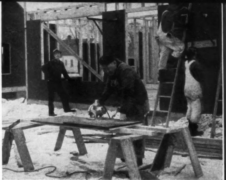
SAWING insulating sheathing with a power tool is 5 times faster than when done with a hand saw, thus helping reduce building cost.
