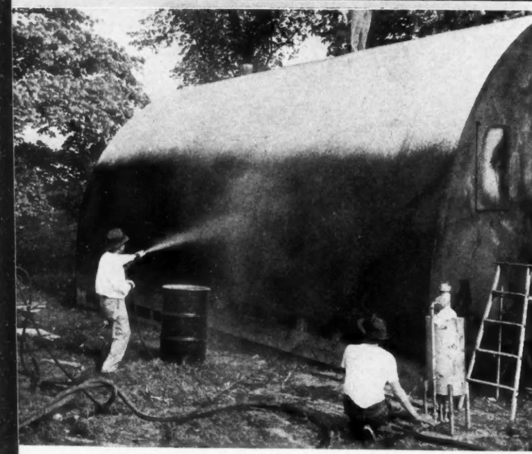
STEPS in building the Purdue war worker's house; top, curved-rafter and trussed-joist frame; middle, gypsum board is nailed on; bottom, waterproofing asphalt is sprayed on, to be followed by paint.
