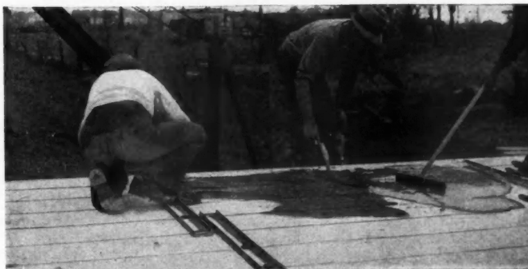
Grout is worked into joints to form mortar key as soon as channels have been placed.
