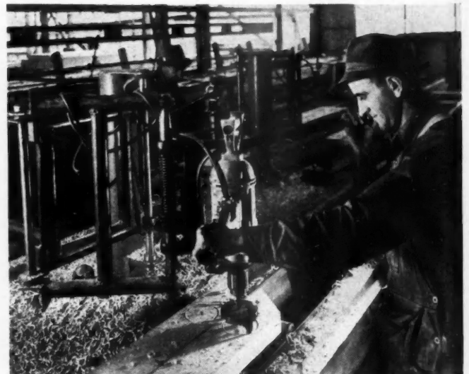
CUTTING split ring grooves at fabricating plant. Note radial actung frame which holds drill for convenience in spotting bolt holes.
