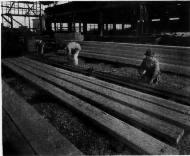
MARKING location of bolt holes using template equipped with special punches which automatically spring back after being driven.
