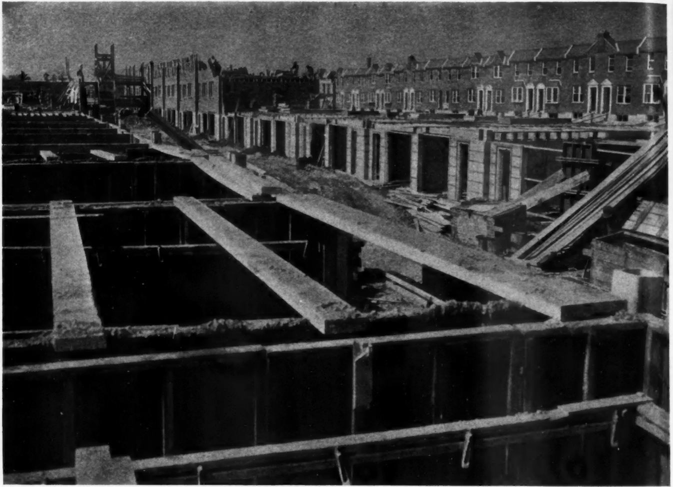
PLYWOOD FORMS used by A. P. Orleans as he speeds another two streets of row houses for Philadelphia war workers. This striking progress picture shows various stages which was started in February. Advance sales totaled 180 in three weeks.
