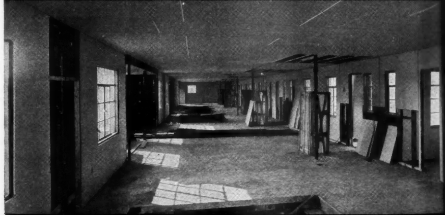
Walls and ceilings of a typical five-room house have been finished in as little as 40 man-hours. 100% salvage in demountable units is possible.
