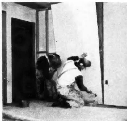
Putting Mengel Bord sheets in place. Edges glued to strips on stud.
