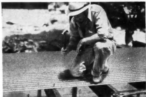
Nailing corrugated sheets to Stran-Steel floor joists. This forms a working deck during the early stages of construction. Later, concrete will be poured over the metal sheets, forming a safe, silent, fireproof floor.
