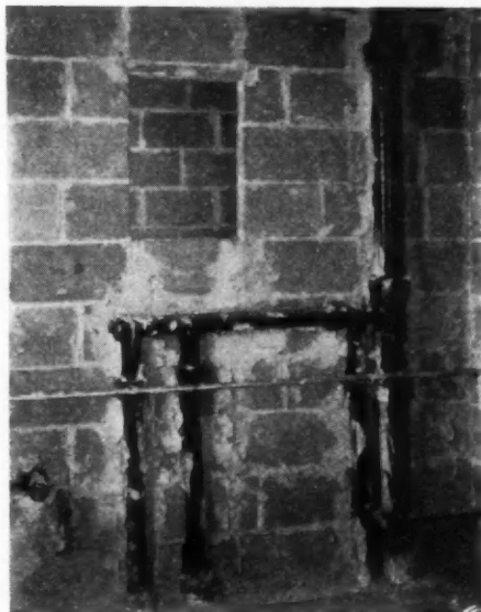
SHOWING interior block partition between kitchen and bath; note compact, roughed in plumbing.
