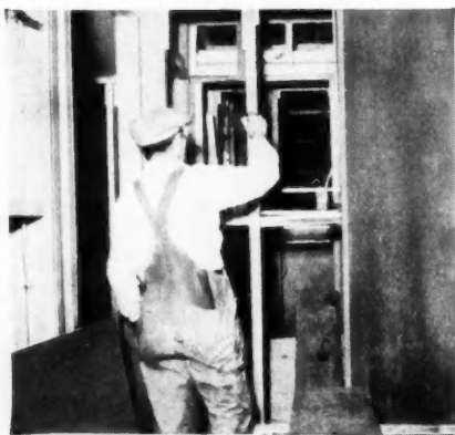
Applying glue to Mengel Bord strips on studs, before installing Mengel Bord sheets.
