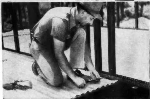
Studs are secured to bottom plate with self-threading screws. Notice that studs (and floor joists) are placed 24 inches o.c. This wide spacing is possible due to the great strength of Stran-Steel—results in savings of material.
