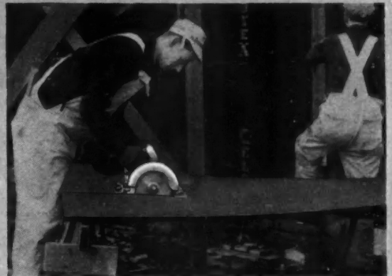
INSULATION MATERIAL being cut to size right on the job, with Black & Decker No. 85 Quick Saw. These fast saws cut lumber, compositions, tile and stone.
