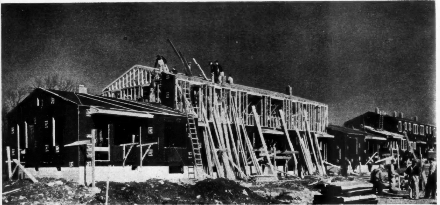
ARMY MEN'S FAMILIES will live in this 6-family apartment under construction at Fort Devens, Mass.; C. J. Maney, Inc., builder.
