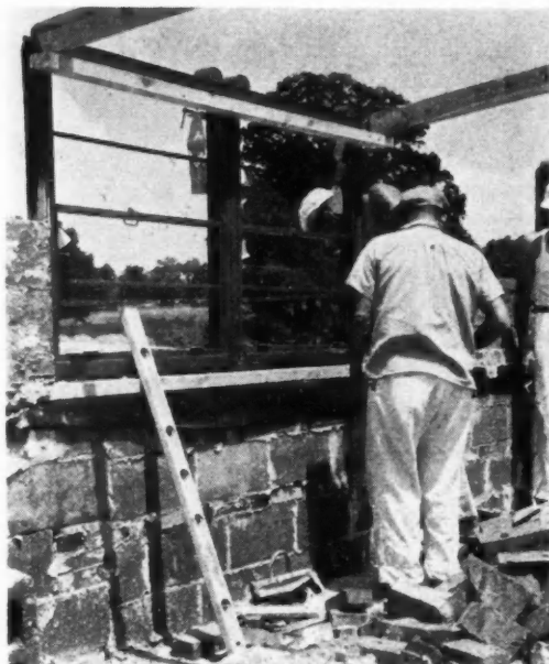
NO TIME WASTED on Marling job as modern type double-hung steel windows are set into masonry walls.
