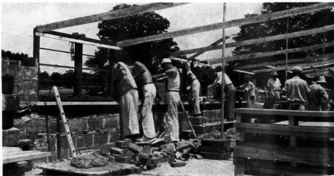
DOUBLE-HUNG STEEL WINDOWS set in place as masonry crew rushes Marling homes to meet demand. Note waterproof membrane strip which has been set in place below windows.
