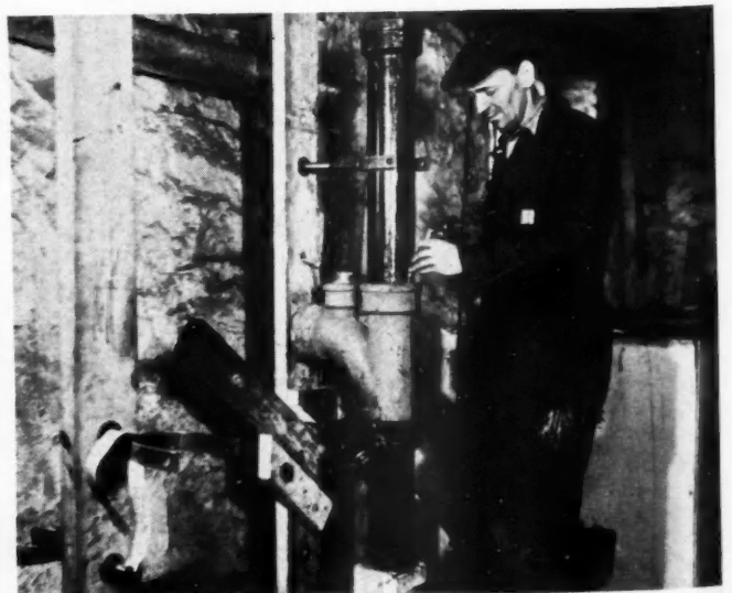
PLUMBING STACK sub-assemblies are made up in the shop and quickly installed on the job at considerable saving of time.
