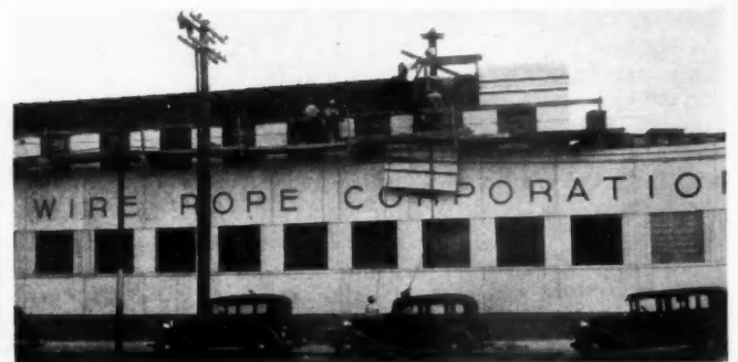
MODERNIZING a large industrial building with architectural concrete slabs made with Atlas White cement. Note shape, thinness and large size of the panel being moved into place.
