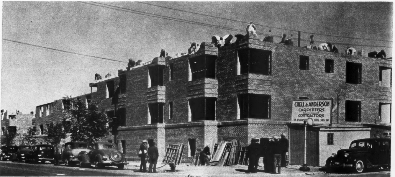
HOYNE-GRANVILLE APARTMENTS under construction in Chicago by Chell & Anderson, carpenters and contractors, financed under FHA plan.
