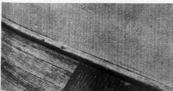
EXPENSIVE TRIM is practically eliminated in the Alden homes. Detail above shows junction of floor with wall, using simple three-quarter round. FLOOR PLAN AT RIGHT SHOWS MODEL FLOOR PLAN WITH ATTACHED GARAGE AND A COMPACT ROOM ARRANGEMENT.
