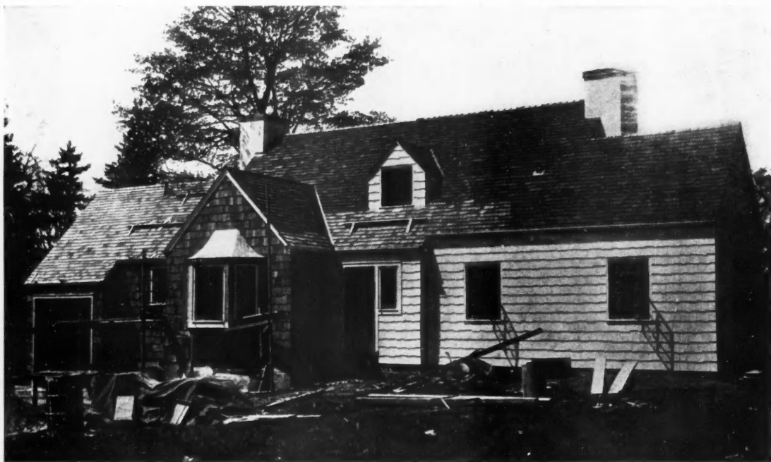
CONSTRUCTION VIEW of colonial cottage pictured on opposite page. Photographed May 11. Four of this type are now under construction.
