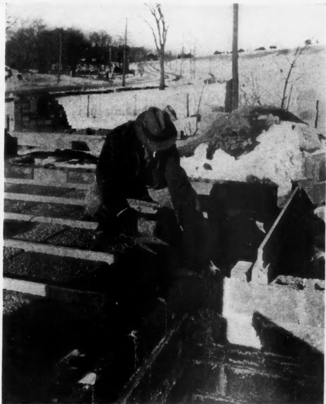
CINDER CONCRETE FLOOR SLABS being placed between precast concrete joists by builder.
