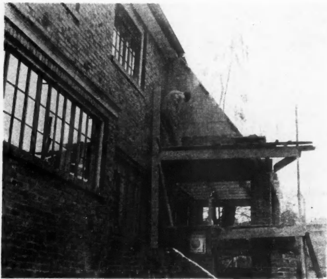
CONSTRUCTION OF ADDITION in progress, showing workmen applying reinforced steel mesh for concrete backing of face brick
