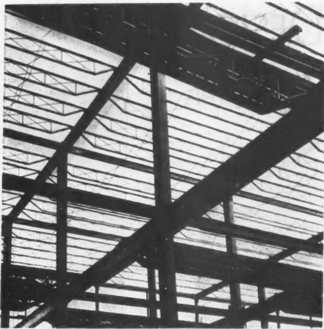
LIGHT WEIGHT STEEL TRUSSES used in construction of Travel and Transport Bldg., World's Fair. Trusses are produced from special I-beam blanks by hot slitting and rolling process, are made in all lengths up to 32 feet. Cord and web members are one piece. Joists are used in combination with a concrete slab and plastered ceiling for light-occupancy buildings, such as apartments, hotels, schools, residences—Kalman Steel Corp.
