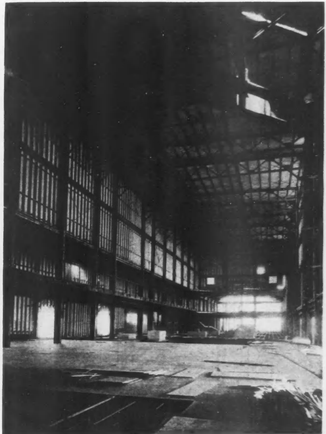
HALL OF SCIENCE—interior showing structural work and laying of plywood floor in large sections. Plywood panels with shi lap edges providing tight joint were also used on exterior.
