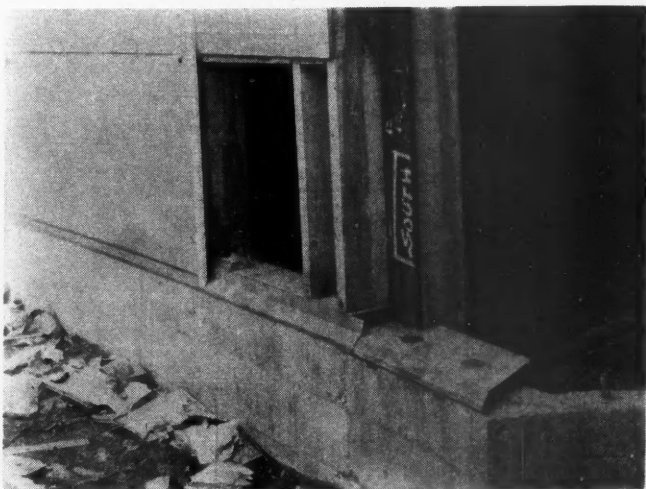
Detail of exterior wall showing application of gypsum board. Metal strip is attached to bolted plate
