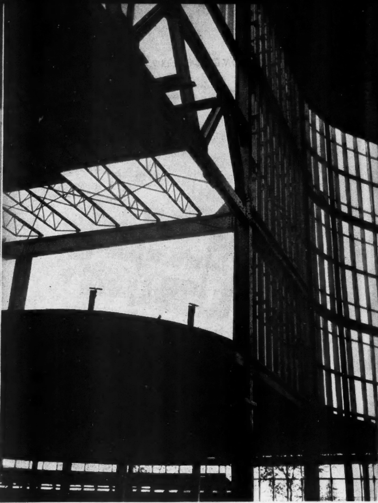
2—General Exhibits building showing wall and roof framing. Roof decking partly in place.
