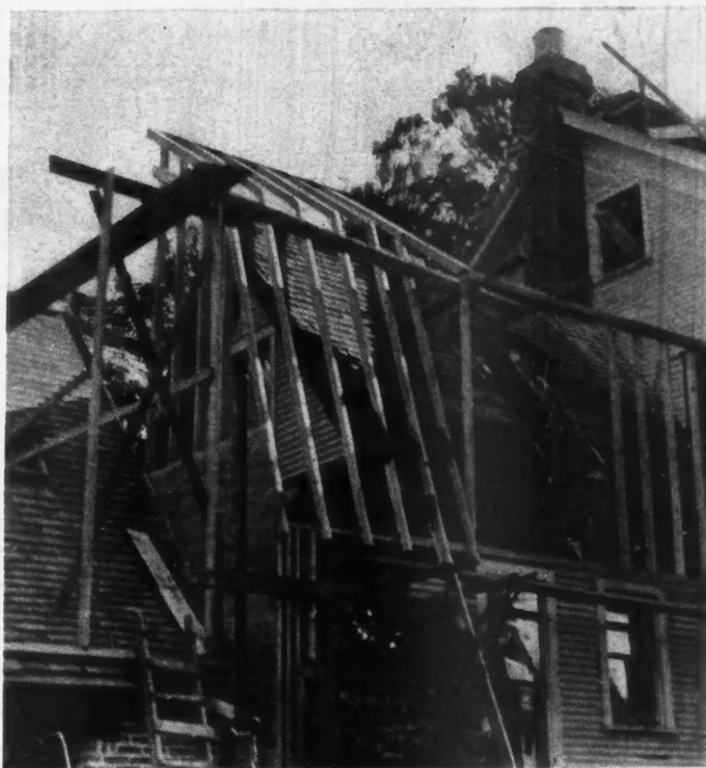
Building up the rear of the house and extending it to connect with new garage at left.
