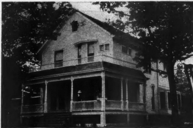
How the Watkins residence looked before the work was started. It was a burden on the owner.
