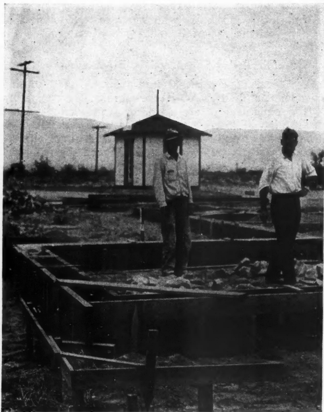
2" PLANKS USED in forms for concrete foundation to be reused later as floor joists. P. G. Owen, Contractor (at right), says forms are easy to build and brace.
