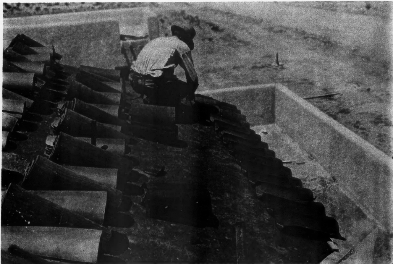
THE STARTING COURSE of a Capistrano tile roof, showing method of laying-off and figuring overhang. Tile is laid twenty per cent random, over ten-year guaranteed composition roof, W. E. Rudasill, Builder.
