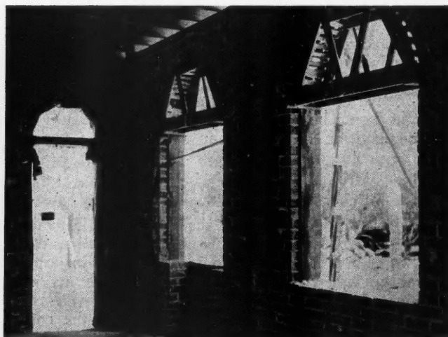
CENTERING FOR BRICK arches over door and windows, solid brick wall construction as employed by Herbert F. Brown, Tucson, Arizona, Contractor.
