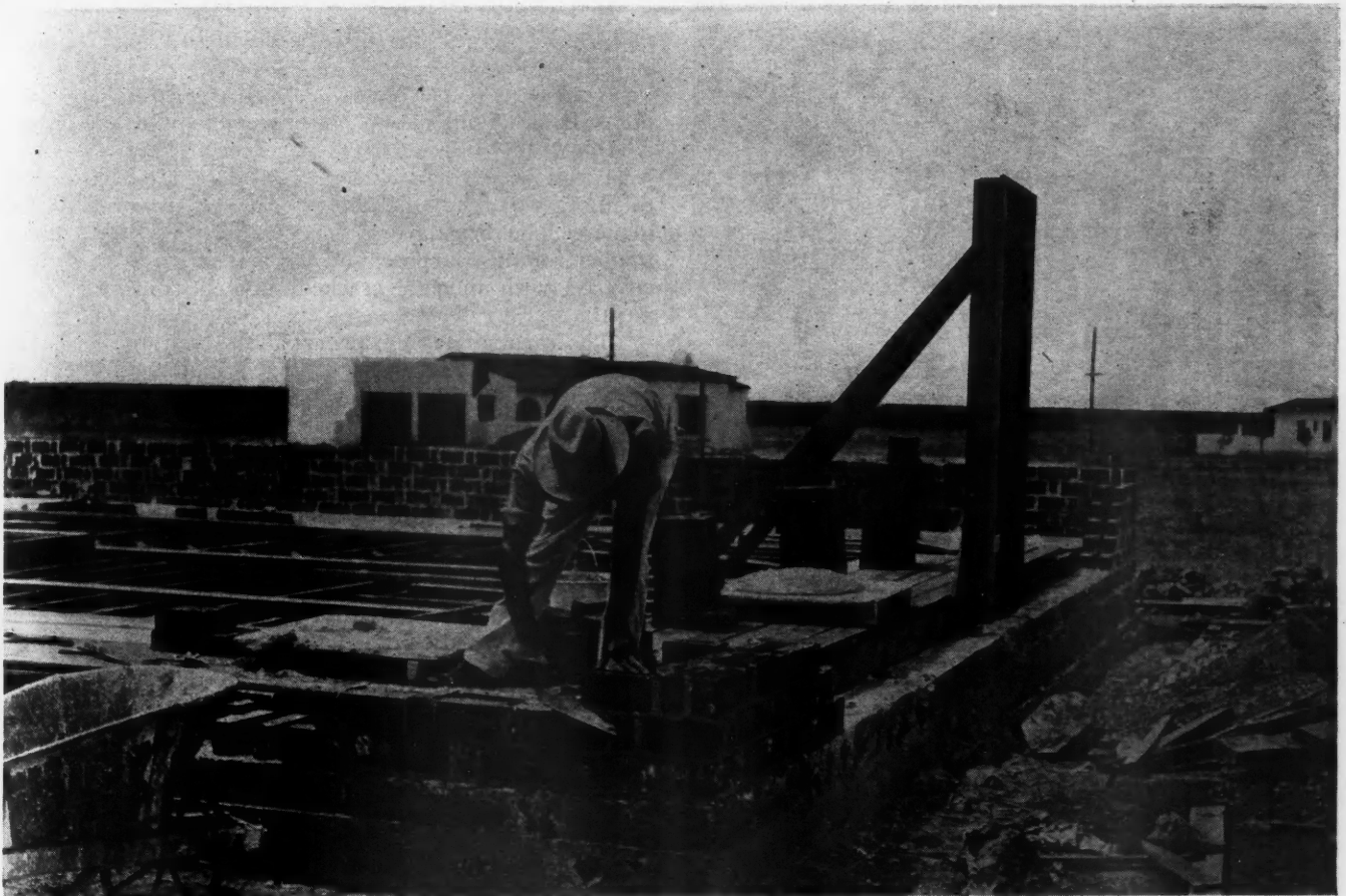
IDEAL BOND , brick wall construction popular in southwest. Glenn Kaiser, brick contractor, demonstrates corner layout. Large size brick 3x4x8 \frac{1}{2} "', run 81 to square yard for nine-inch wall; leaving air space in center.
