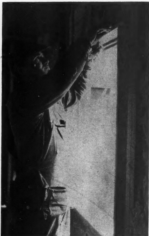
The Various Mineral Wool Materials Are Often Applied by Hand and Can Be Tucked Into Every Crack and Crevice Around Openings.
