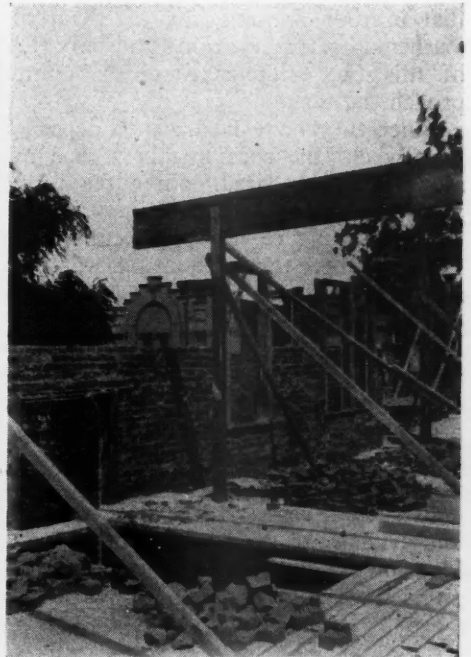
Beam Supported at End, Rubin & Cohen. At Left Below: John Grandy, San Francisco, on Job with Photographer
