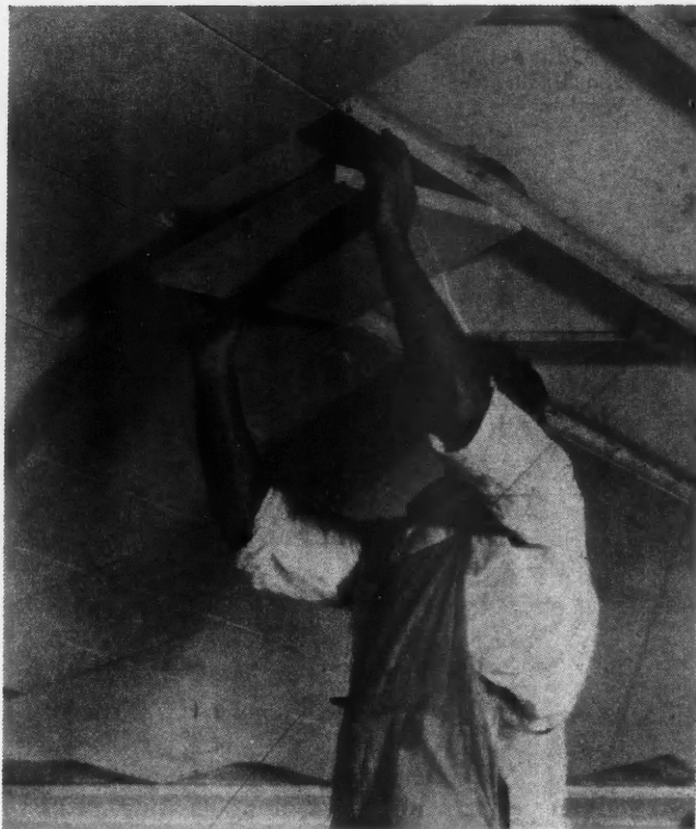
Perforated Metal Tile, Filled with Sound Absorbing Material, Are Used for Acoustical Correction, and Permit Painting or Other Decoration.
