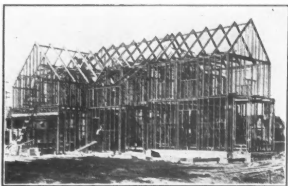
The twelfth day after operations were started. Steel Frame completely finished ready for the stone work
