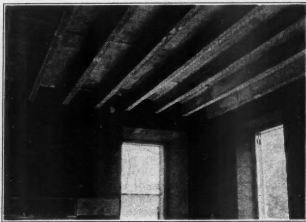
Hangers Imbedded in the Concrete Joists Provide a Means of Attaching Metal Lath to Which Plaster for Ceiling Is Applied.
