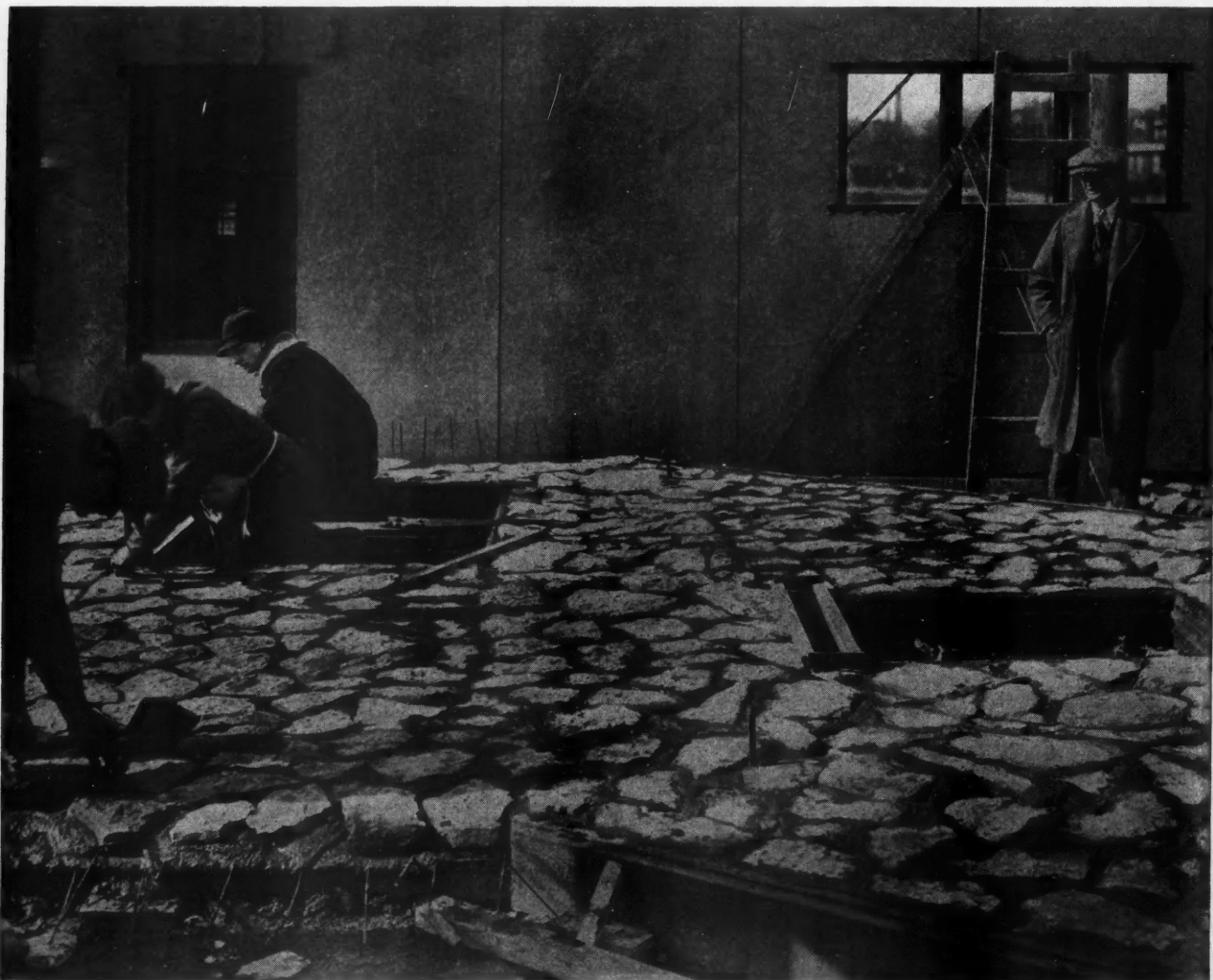
In the Foreground, Unskilled Workmen Are Embedding Stone Slabs in the Soft Mortar to Make the Outside Decorative Face of One Side of the House. In the background we see the inner face of the adjacent side wall, already raised.
