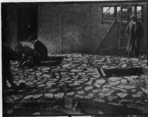
The photo above shows how Tri-Ply walls are built lying on a flat surface.
