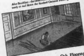
After breakfast—the room cleared and the carpenter ready to nail down the finished CROMAR Flooring
