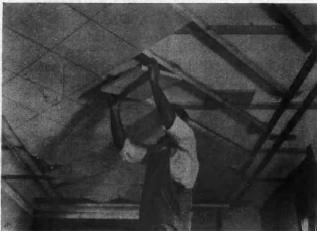
These Tile Are Attached to the Ceiling by Inserting in Metal Tee Stripes Which Lock Them Rigidly in Place.
