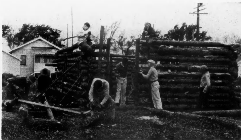
Scout Troop 27, of Sacramento, California, Building a Log House as a Part of the Better Homes Celebration. This troop also built a primitive grass hut and an Indian tepee, showing the evolution of the home.
