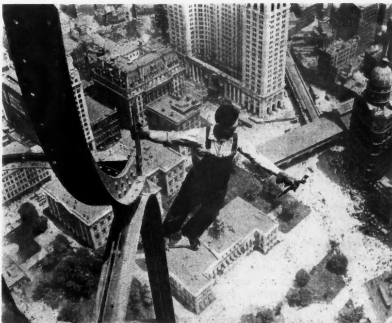
This Picture Shows Clearly the Kind of Foothold on Which Structural Steel Men Must Rely. It must be exhausting work to hang on with one hand and work with the other, yet the men of the steel crew frequently do it.
