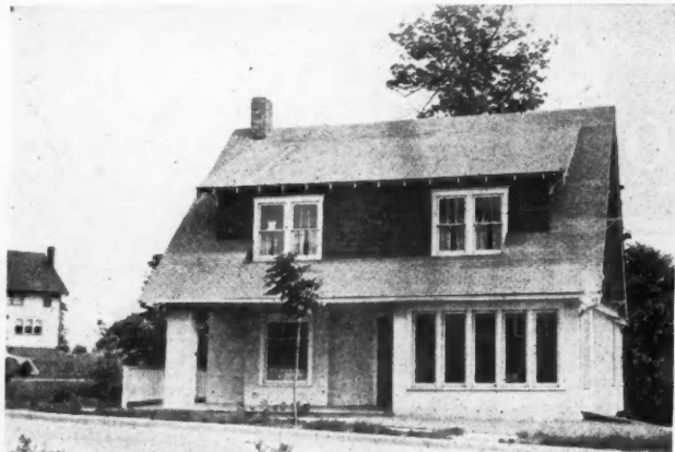
Fig. 5. An Otherwise Neat Stucco House Badly Discolored Around the Base Because of Being Too Low.
