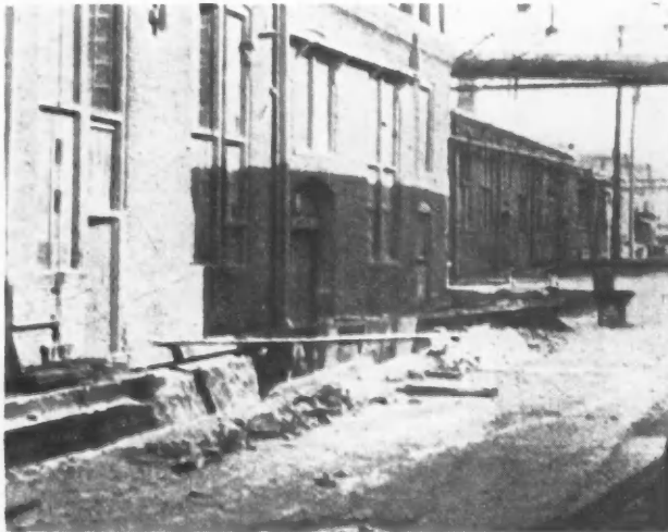
By the Use of Minimum Charges, Spaced Close Together, a Foundation May Be Blasted Without Danger to Adjacent Buildings.
