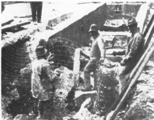
Woven Wire Fencing Will Serve as a Blasting Mat to Protect Nearby Objects Which Might Be Injured by Flying Pieces of Concrete.
