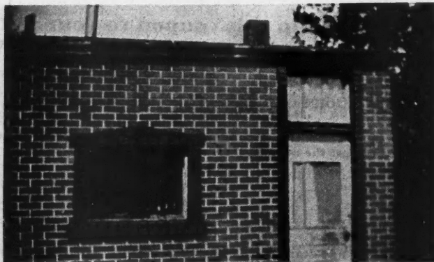
A Stucco Wall Finished with the Aid of a New Device Gives a Very Satisfactory Imitation of Brick.
