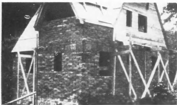
This House Under Construction Shows the Rough Wall Built of the New Fibrous Block.
