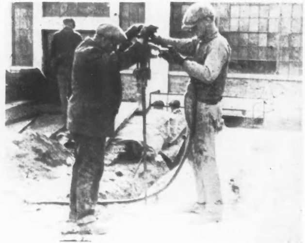
If an Engine Bed or Similar Foundation Is to Be Removed the Holes May Be Drilled Vertically and the Charges Fired One at a Time with Cap and Fuse.
