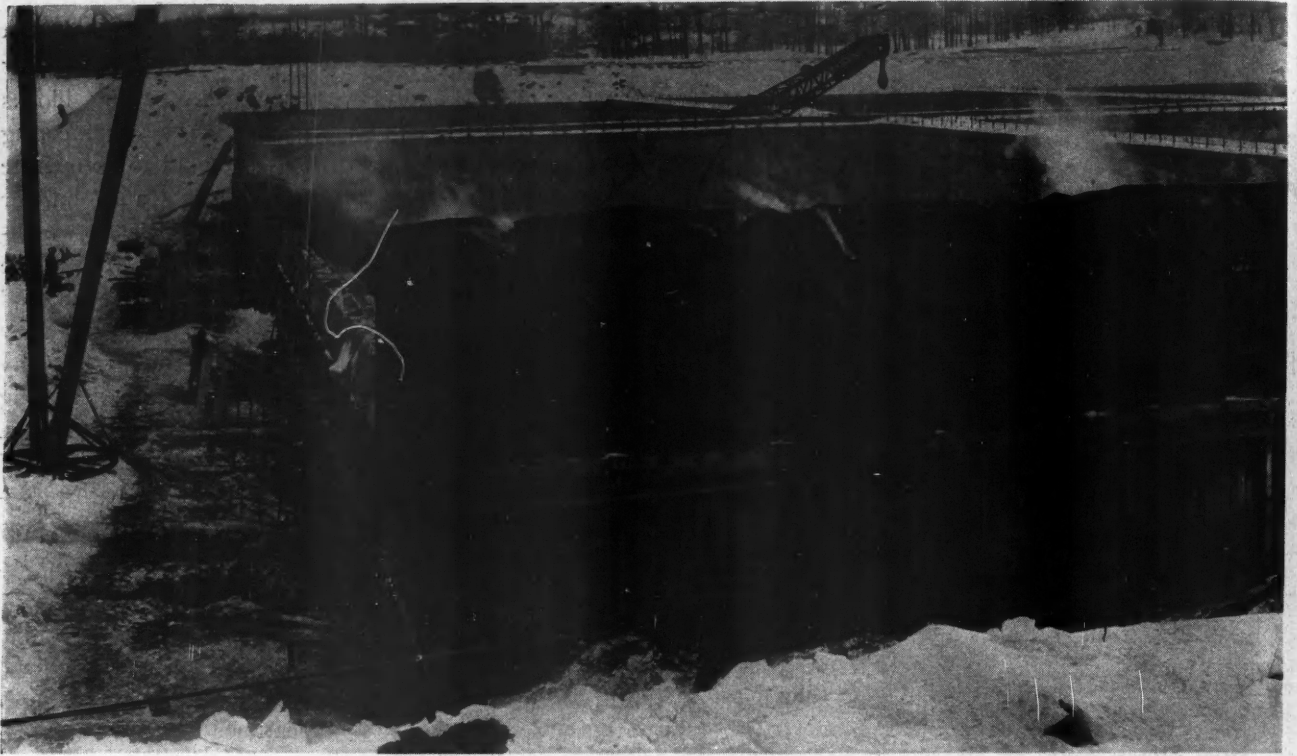
In Winter Concrete Construction the Contractor's Profit May Depend Largely on the Progress He Can Make Between the Temperatures of 32° F. and 18 or 20° F.
