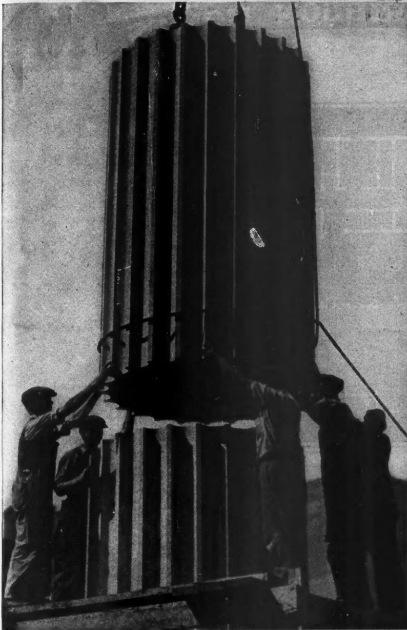
Some Hoist! Some Lift! Easing one of the 25-ton granite columns into place for the new court house, New York City.
