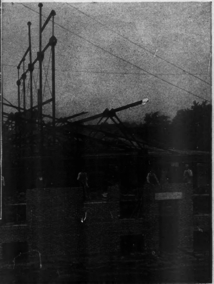
The Wholesale Poultry and Egg Storage Plant as It Appeared Under Construction. The builder was able to go ahead with absolute certainty of his work and without delay, being helped by plans furnished him from the maker of structural steel frame and lumber. It made a fine job and brought him many others.
