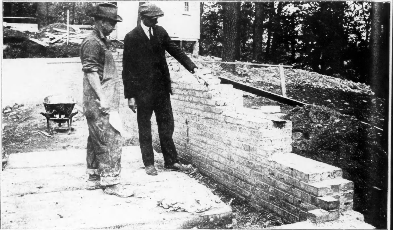
The World's Most Perfect Home is being built in Glen Ellyn, Ill., a suburb of Chicago. Brick solid foundation and walls.
