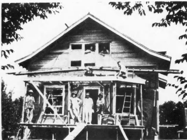
Builder Reed Keeps Himself and Employees Busy Erecting Substantial Dwellings of This Type in Iowa.
