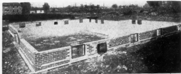
Fig. 2. More Windows Are Installed in Basements Since the Steel Frames Have Come Into Use. This single home provides for thirteen.
