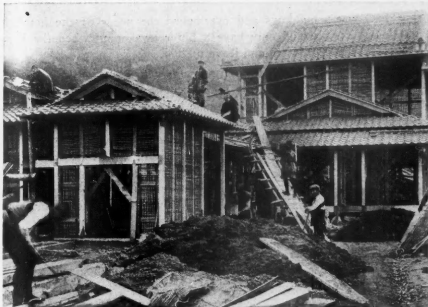
Putting the Finish Touches on Homes in Japan. The Roofs of the Houses Are Covered with Roof Tile.
