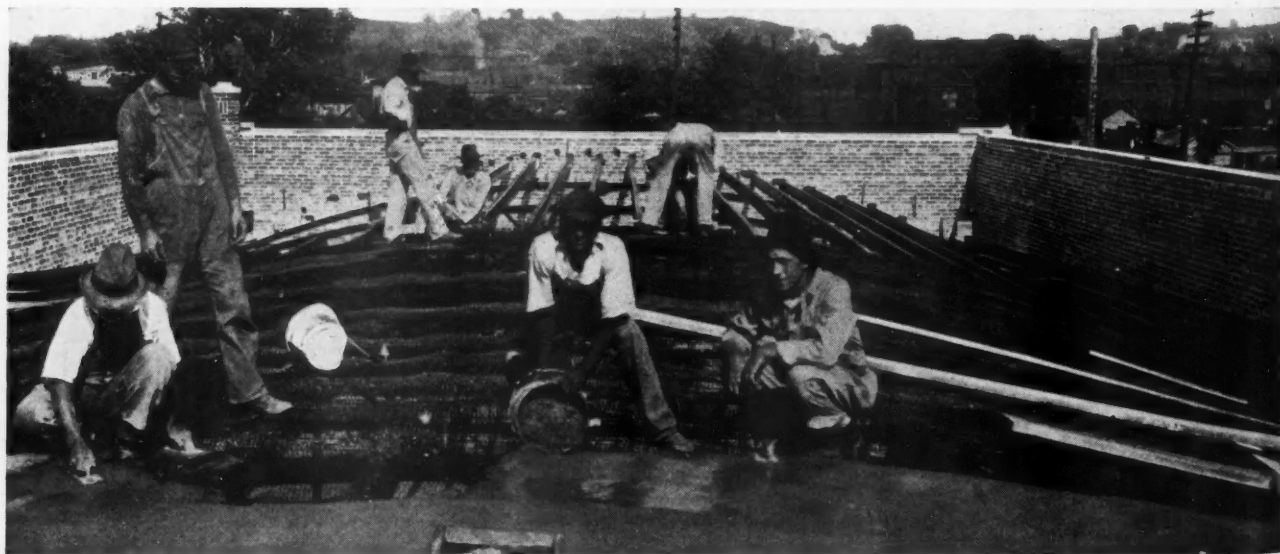
Workmen Spreading Cement Roof on Metal Lath Supported by Steel Lumber Joists Resting on Structural Steel Truss. The Metal Lath Is Clipped to the Top of the Joists as Centering for 2-Inch Concrete Floors and Roofs and Clipped to the Bottoms for Coat of Plaster.
