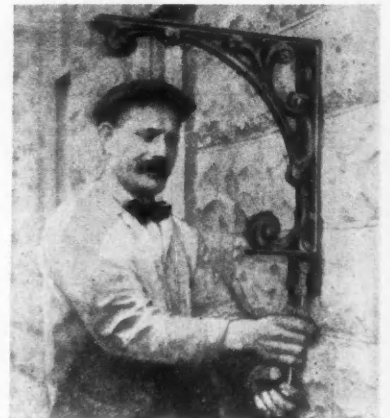
The Bracket in Place. The Workman Is Now Tightening Up the Expansion Bolt. Each Turn of the Bolt Spreads the Interior Shell and Increases Its Grip on the Wall.
