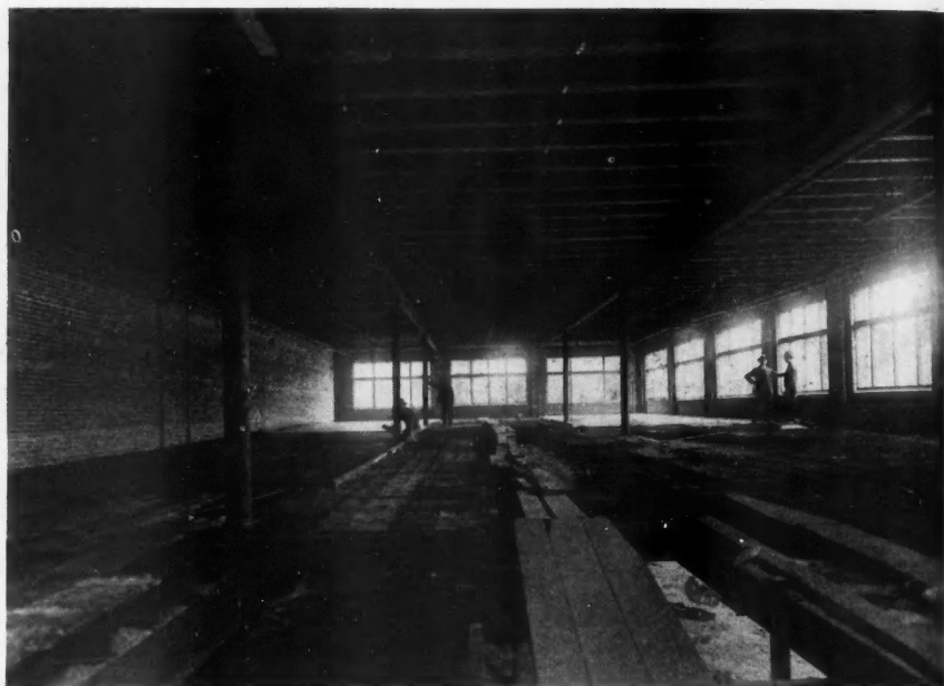
Interior William A. White Garage, Emporia, Kan., Showing Steel Lumber Joist Floor and Roof Construction Supported on Cast Iron Columns and Structural Steel Beams. It was Designed by W. F. Marx, Architect, Emporia.
