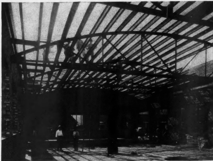
Curve Roof Garage, St. Joseph, Mo. The Light Structural Steel Trusses Are Supported on Brick Bearing Walls with Steel Lumber Floors and Roof.
