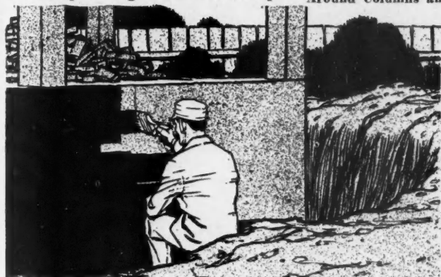
This Shows Foundation with the Dirt Thrown Back, so That Waterproofing Paint Can Be Applied to the Whole Surface of the Wall from the Footer Course up to the Grade Line. The Top of the Footer Course Should Be Coated with Waterproofing Paint Before Foundation Walls are Placed Upon Them.
