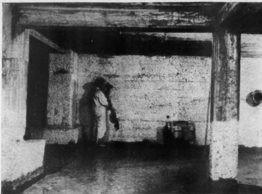
Surface Under Course of Preparation for Application of Waterproofing. The Entire Face Is Removed to Expose the Aggregate. Note the Method of Carrying Waterproofing Around Columns and Pilasters.
