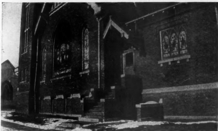
Close-up View of Church Door Leading to Lecture Room and Basement. The Rector Wants to Enclose the Entrance to Protect the Rooms from Rain and Snow.
