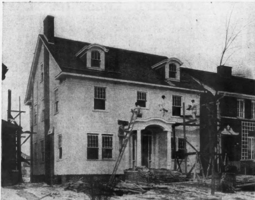
Winter Did Not Stop This Stucco Job. Robt. W. Speedie, Contractor in Detroit, Believes in Living Up to the Significance of His Name. He Tackled This Work in Dead Winter and as a Result the House Was Ready for Its Owner in Early March Instead of the Usual May.
