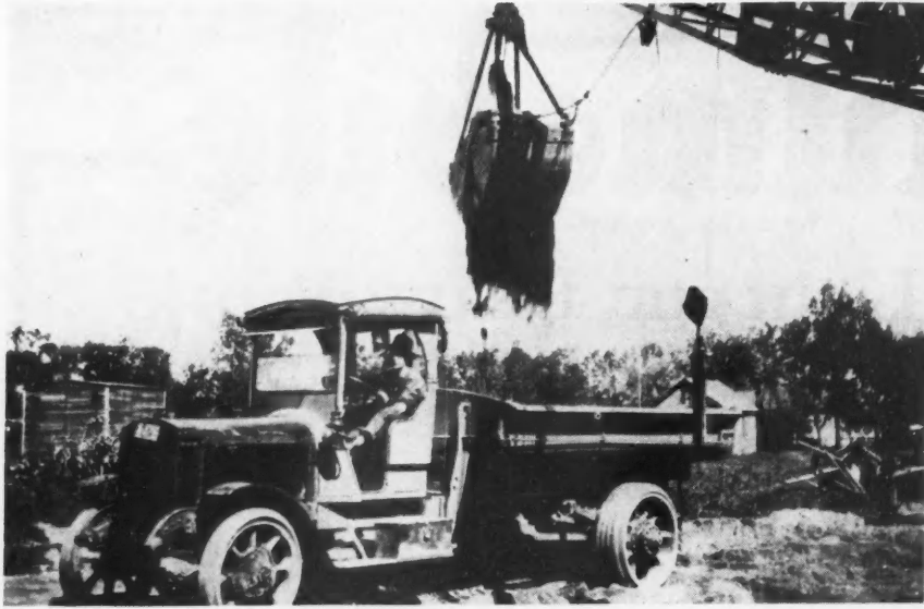
One of the Two 5-ton "Acme" Trucks Used on the Excavating Job by the S. J. Peterson Co., Minneapolis. The Camera Was Snapped Just as the Clam Shell Was Releasing Its Load.
