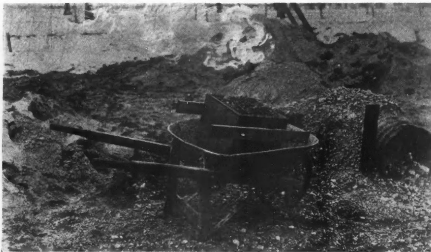
Showing How Corrugated Steel Culvert Pipe Is Used as a Heater for Concrete Materials in Freezing Weather.
