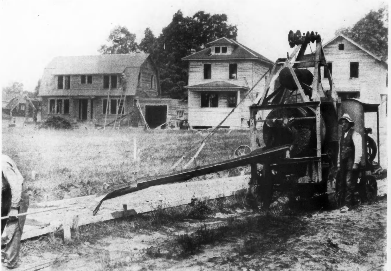
W. A. Leyrer, of Lansing, Mich., and the Paving Mixer Which He Has Adapted to the Work of Laying Concrete Sidewalks. Mr. Leyrer Finds the Mixer Saves Time and Labor, Adding to His Profits. He Has Laid as Much as 40,000 and 50,000 Square Feet of Walk in a Day, and Had About Five Miles to His Credit When the Summer Ended. Besides, Mr. Leyrer Uses the Paver to Four House and Other Building Foundations.
