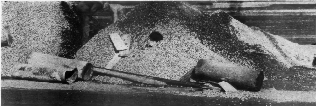
Short Lengths of Steel Culvert Pipe in Which Fires Can Be Built Are Used to Heat Aggregates for Cold Weather Concreting.
