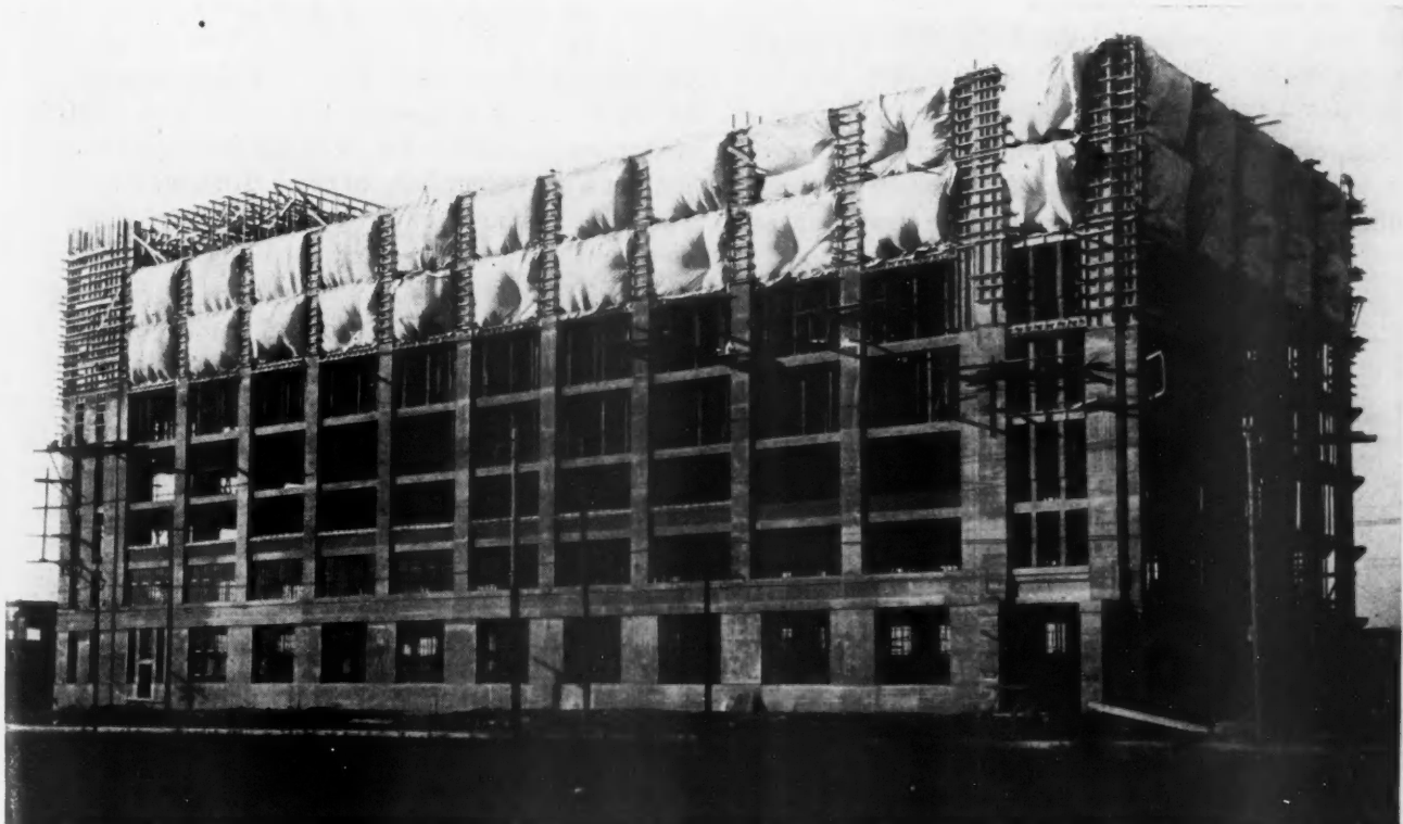
EVEN IN THE EXTREME TEMPERATURES OF CANADIAN WINTERS CONCRETE BUILDINGS ARE ERECTED. The photograph shows a building put up in the winter of 1915 for the Robert Simpson Co., Regina, Sask.
