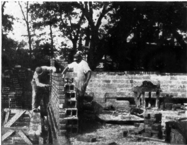
Laying Back-Up Tile and Face Brick Veneer at the Same Time. This Makes a Very High Grade Wall.
