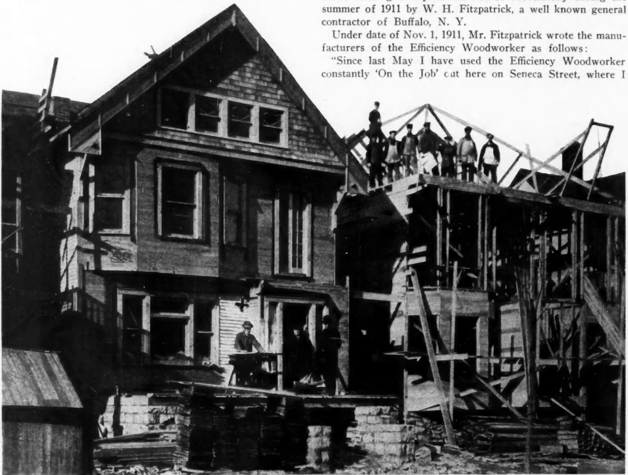
The "Efficiency Woodworker" and Crew at Work on the Last of 40 Houses on Seneca Street, Buffalo. W. H. Fitzpatrick, General Contractor.
