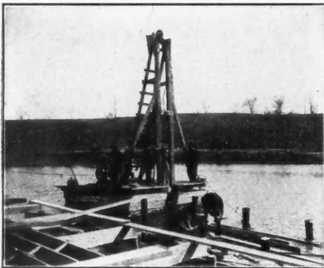
"Sultan" Gasoline Engine and Hoisting Outfit Mounted on a Barge Driving Piles.
