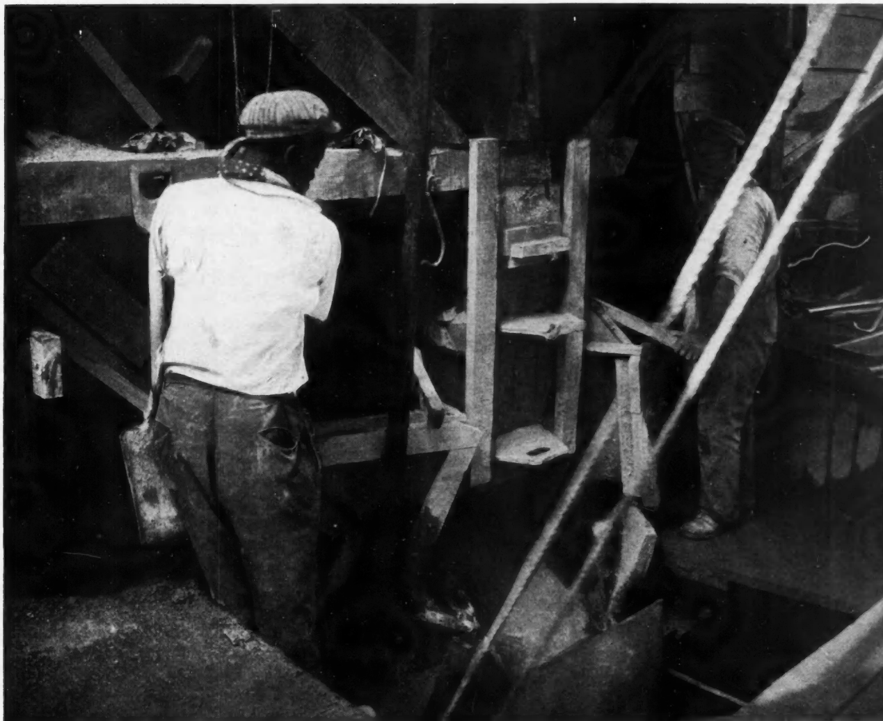
These Two Men Work the Gates That Allow Exactly the Right Amount of Cement, Sand and Gravel to Come Down Each Time into the Mixer. "Let the Teams Do the Work," Says Contractor Weeks.
